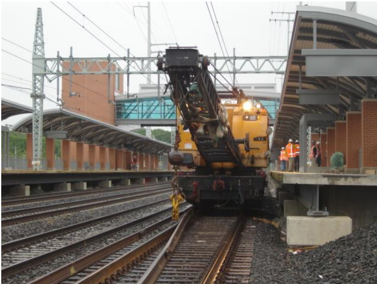
Figure 8. West Haven accident location showing crane position.
