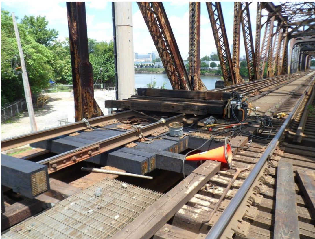
Figure 4. Accident location on railroad bridge with loose grating removed.
