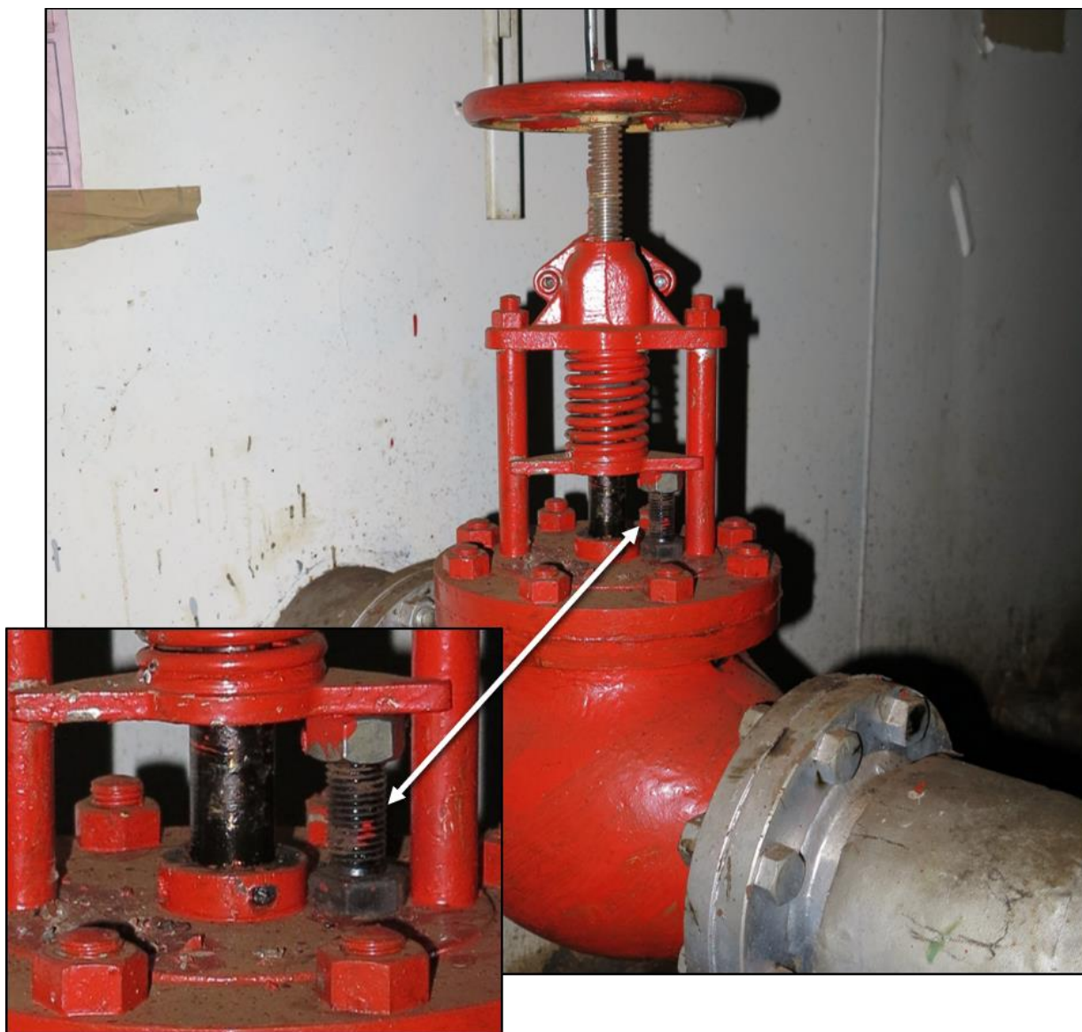
Figure 18. Postaccident photo of Caribbean Fantasy's starboard heavy fuel oil (HFO) storage tank QCV that was blocked open with a bolt and nut.
