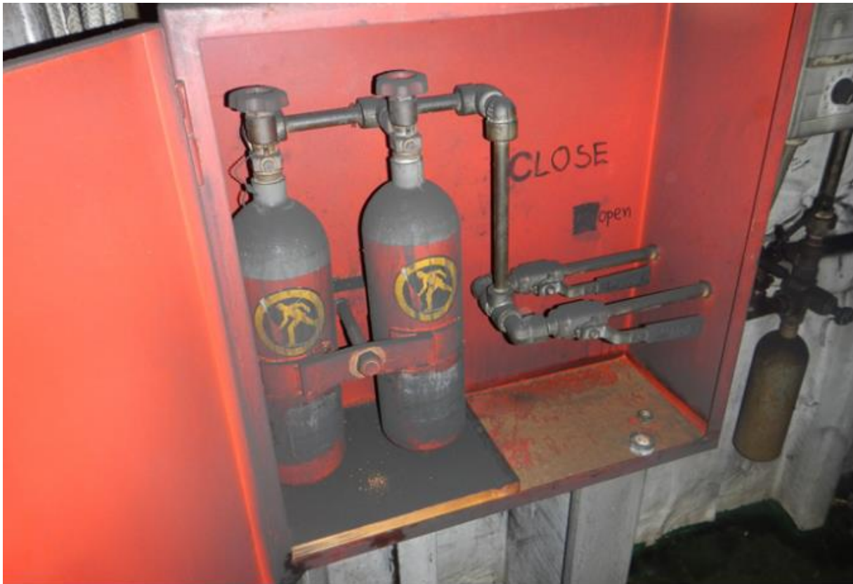
Figure 4. CO 2 system activation station postaccident. Both actuation valves are in the open position.
