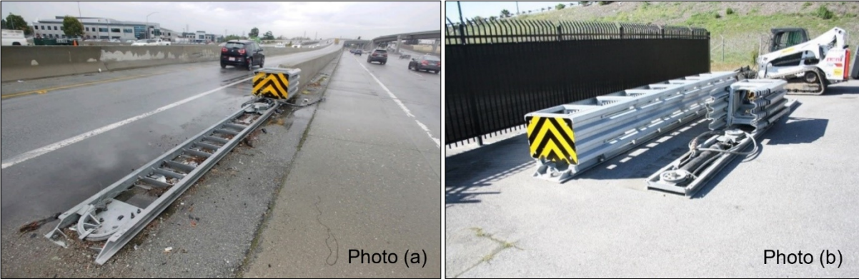
Figure 1. (a) Fully collapsed crash attenuator as it was before the subject crash; it had been damaged during an earlier collision. A Caltrans worker took the photograph on March 20, 2018. (Source: Caltrans) (b) An undamaged attenuator (left) beside the crash-damaged attenuator (right). (Source: Caltrans)
