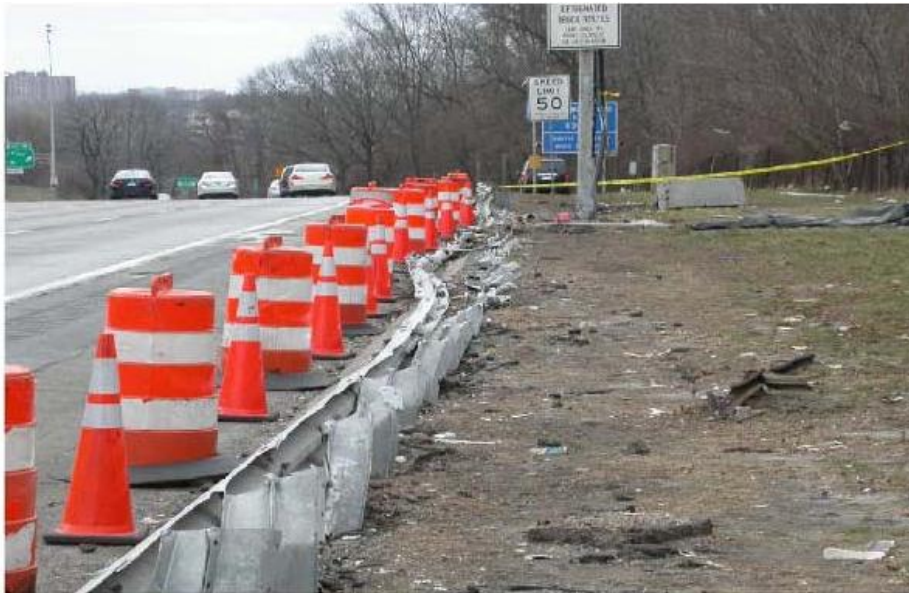
Figure 5. Damaged guardrail at the approach to the vertical highway signpost.
