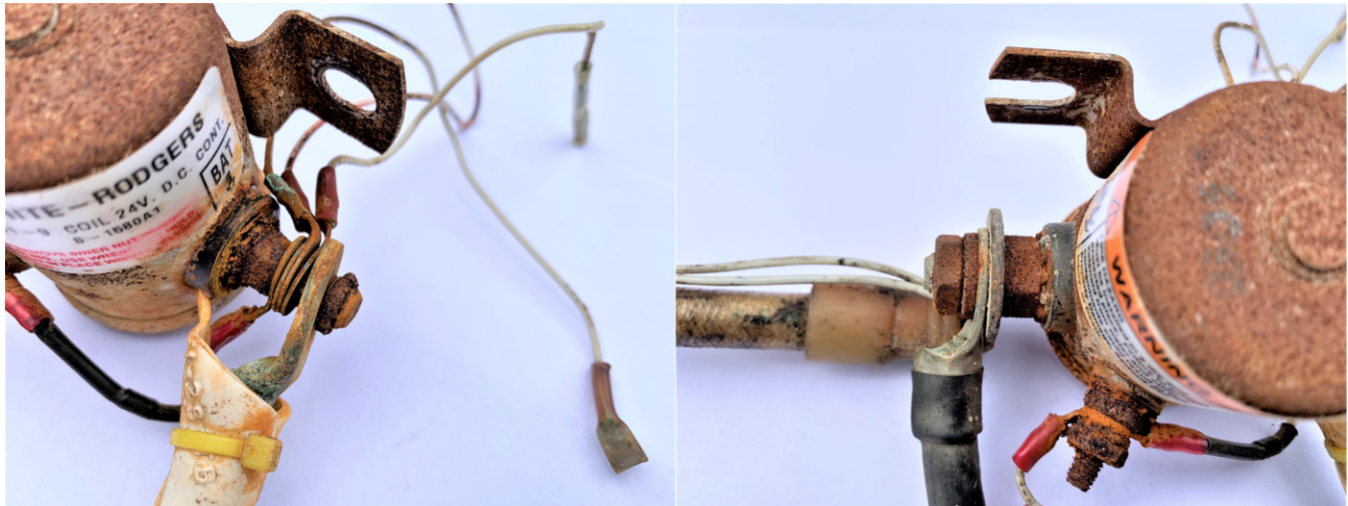
Figure. Battery contactor terminal for the positive battery cable was loose (left). The battery contactor terminal for the battery switch and starter motor contactor cables was tight (right).
