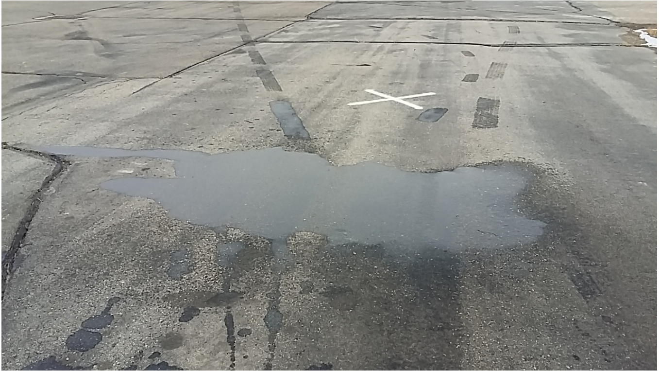
Photo 2 – Oil on Ramp
