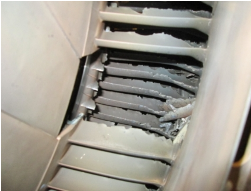
Photo No. 1: View of missing 3rd stage turbine vane cluster from front of LPT. (Delta)
