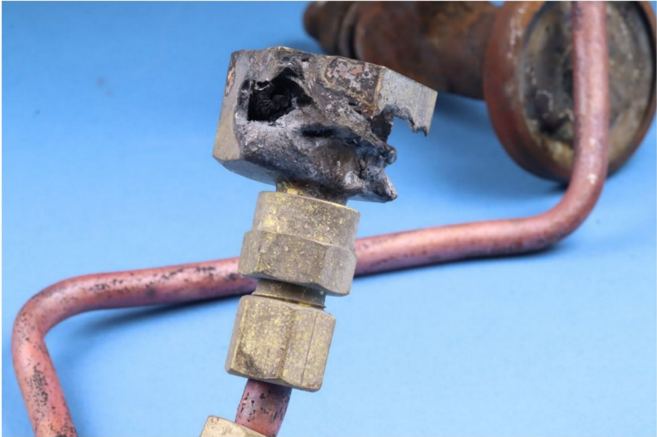
Figure 3. Localized melting of oil pressure line tee fitting.
