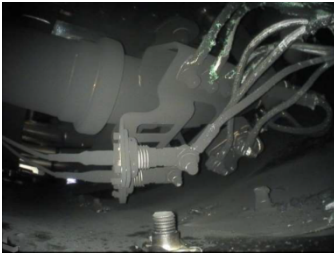
PHOTO 1: SOOTING DAMAGE Photo courtesy of GE
