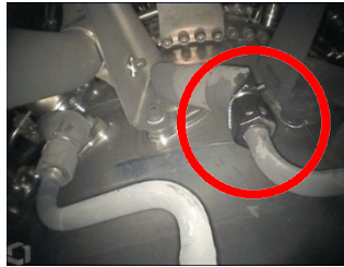
PHOTO 2: FUEL MANIFOLD B-NUT WETTED AT TOP OF ENGINE - POSSIBLE LEAK SOURCE Photo courtesy of GE
