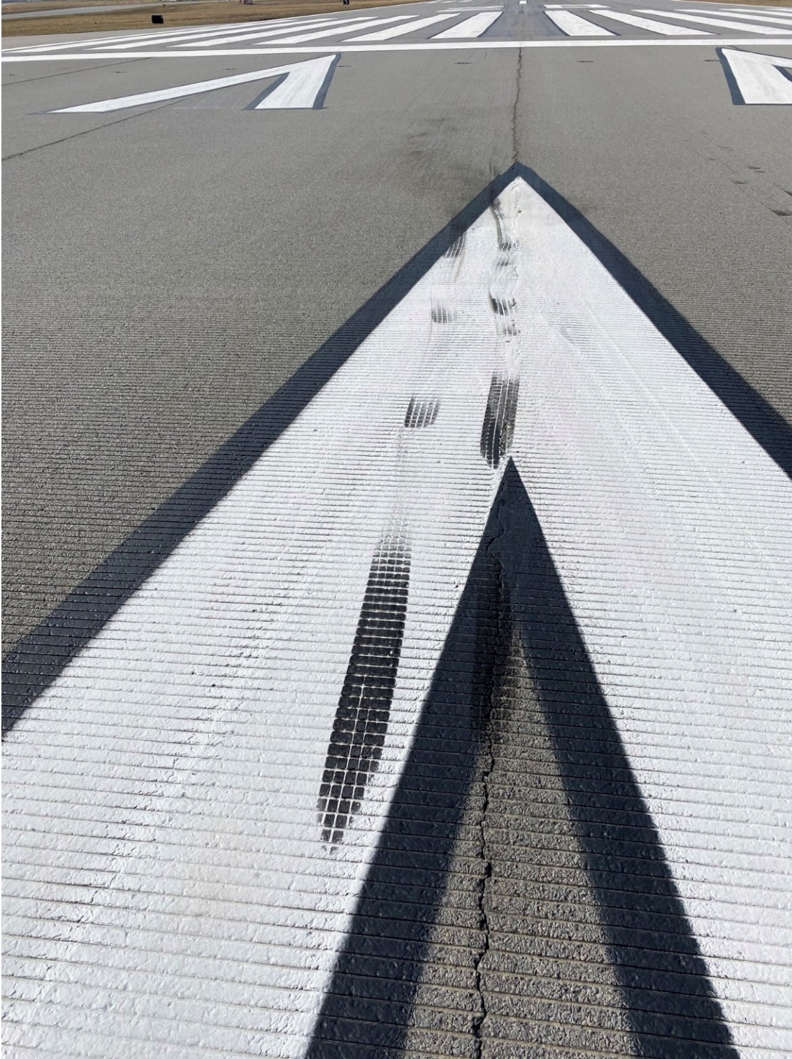
Figure 1 - View of Ground Scars and Rubber Transfer Marks Consistent with Left Main Landing Gear
