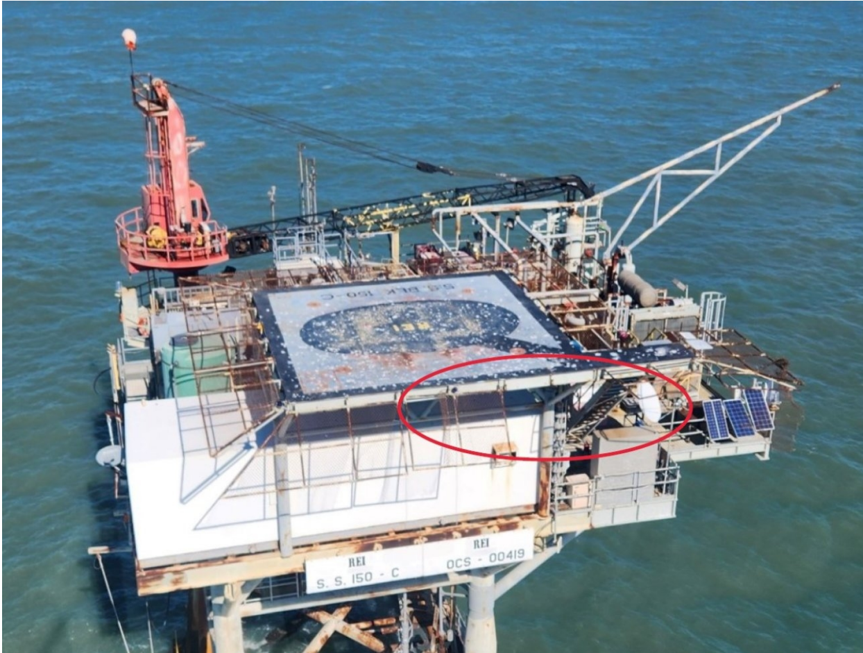
Figure 1. Aerial view of the platform and helideck (courtesy of the helicopter operator). The damaged light and skirting are circled in red at the bottom right side of the helideck near the stairway.
