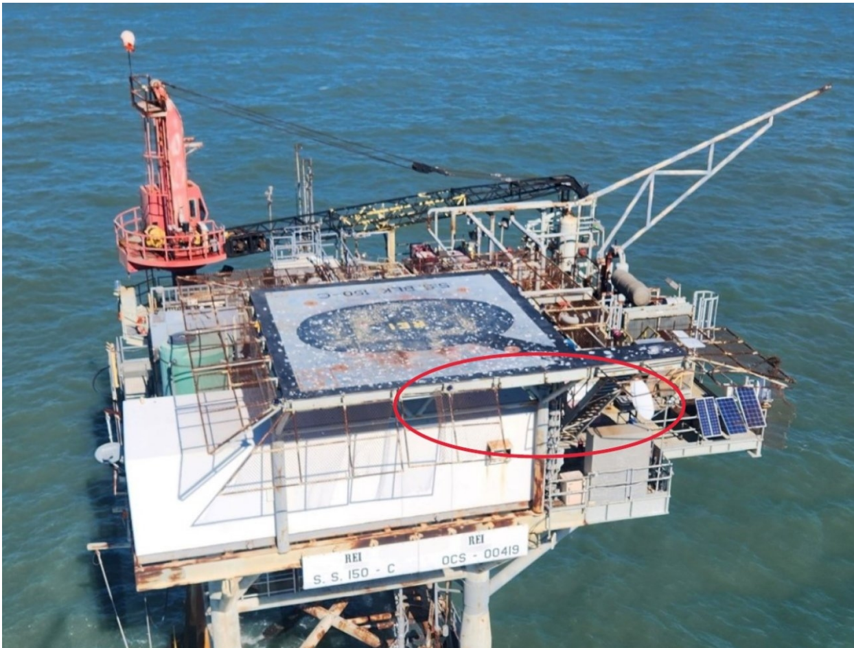
Figure 1. Aerial view of the platform and helideck (courtesy of the helicopter operator). The damaged light and skirting are circled in red at the bottom right side of the helideck near the stairway.
