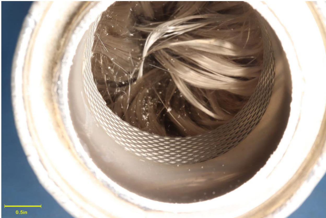
Figure 2. Image of the muffler body inlet, showing the fractured perforated inner tube and the fiberglass packing that had fallen inward.
