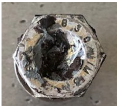
Figure 4. One of the three bolts found on the interior ceiling panels (Source: Swift Air).
