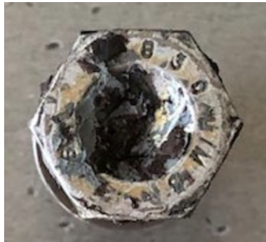
Figure 4. One of the three bolts found on the interior ceiling panels (Source: Swift Air).
