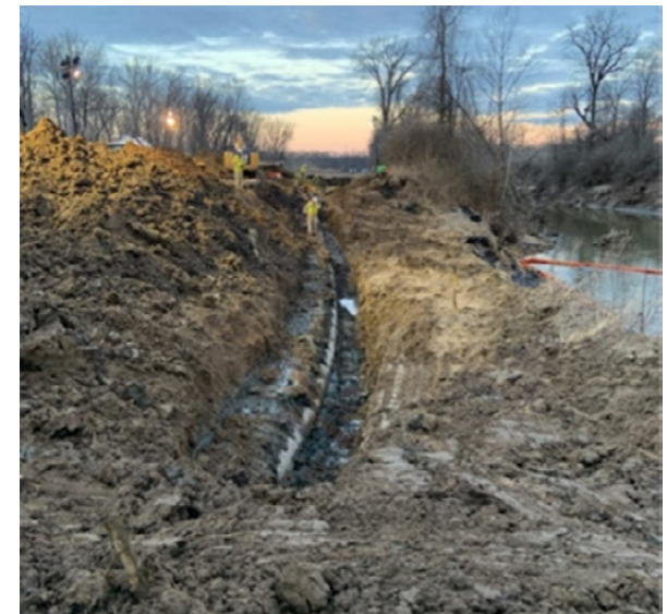
Figure 31. The ruptured Woodpat pipeline, following the release of crude oil into Cahokia Creek, a tributary of the Mississippi River, in Edwardsville, Illinois.
