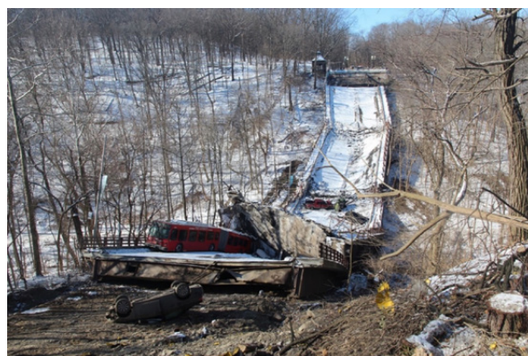
Figure 15. View of the collapsed Fern Hollow Bridge from the east.
