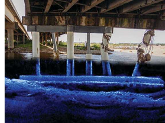
Figure 53. Multibeam sonar images overlaid with above-surface photograph illustrate the damaged columns postaccident (sonar survey taken September 27) on the westbound span of the I-10 bridge. SOURCE: TXDOT
