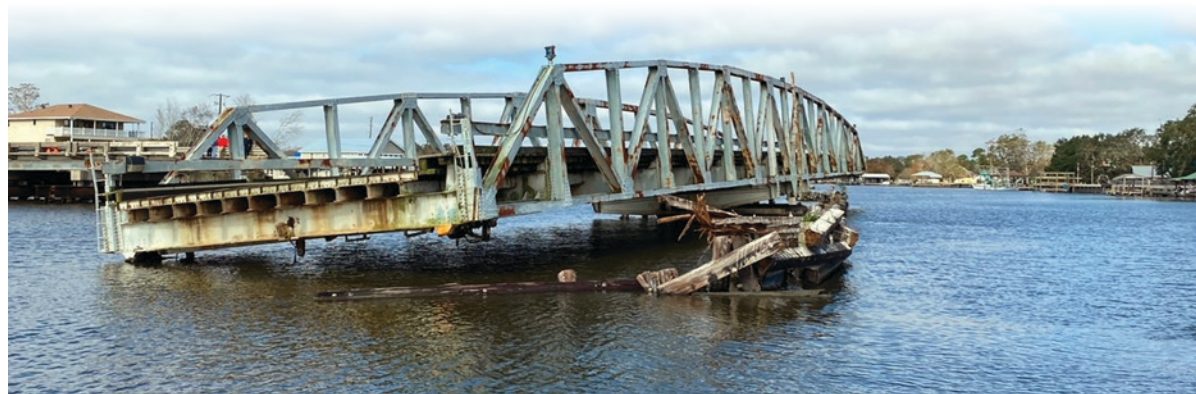
Figure 82. Postaccident damage to Barataria Bridge looking north. SOURCE: ANONYMOUS
