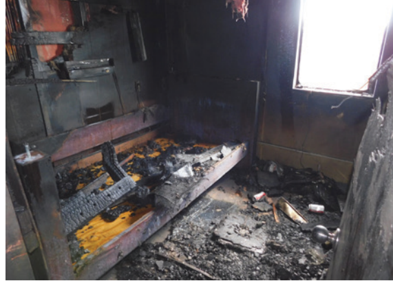
Figure 122. Crew quarters on board the Susan Lynn . SOURCE: LOUISIANA OFFICE OF STATE FIRE MARSHAL
