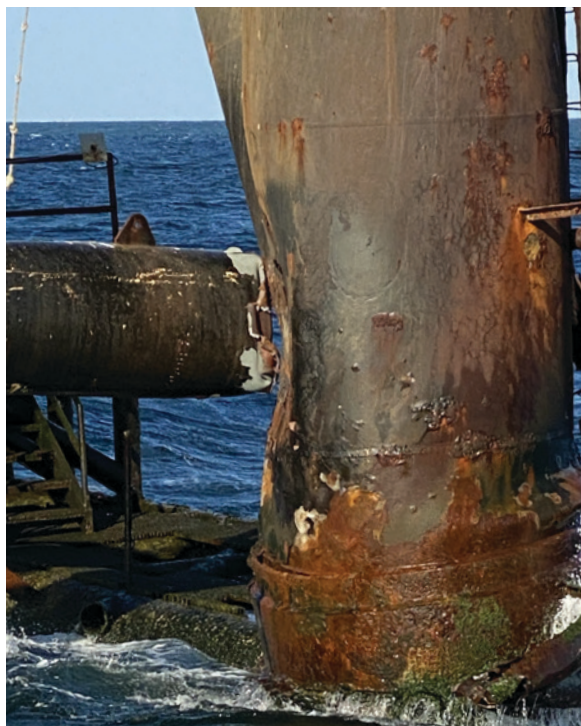
Figure 46. SP-57B's fractured horizontal and damaged leg.
