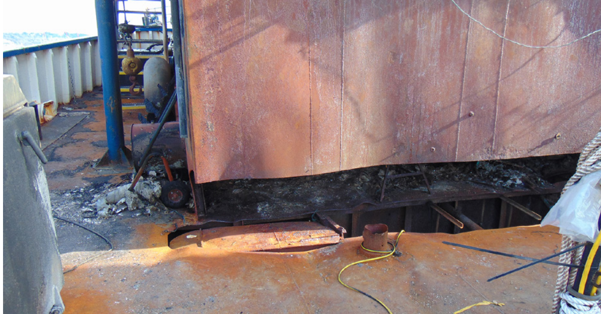
Figure 66. Aleutian Falcon bridge deck post-fire, depicting hot work area on the day of the casualty.
