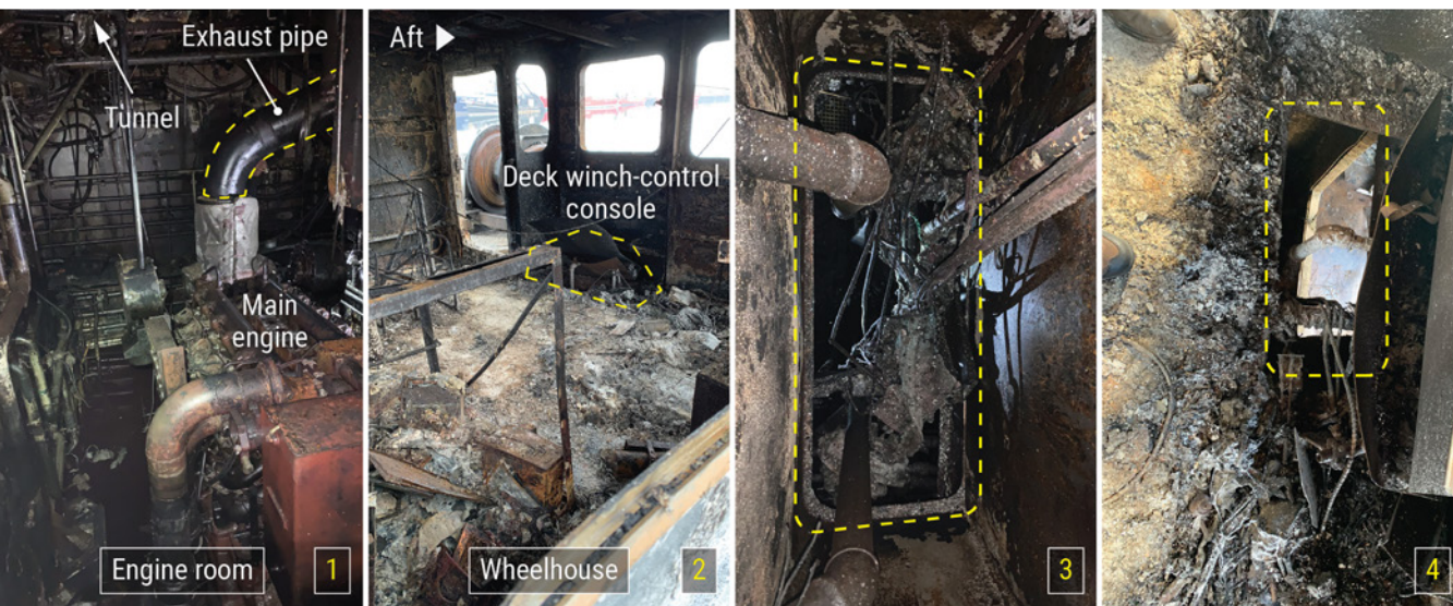
Figure 94. Left to right: Post-fire damage of (1) the engine room, where the crew removed the lagging from the exhaust pipe, as indicated by the dashed line; and (2) the wheelhouse, where the captain observed black smoke emanating from under the deck winch-control console. Damaged pipe/hose tunnel, as identified by dashed rectangles, looking up from the engine room (3), and down onto the deck winch-control console location (4).
