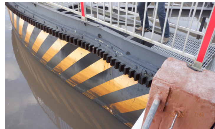
Figure 38. Below: Damaged steel plating and rack on gate.
