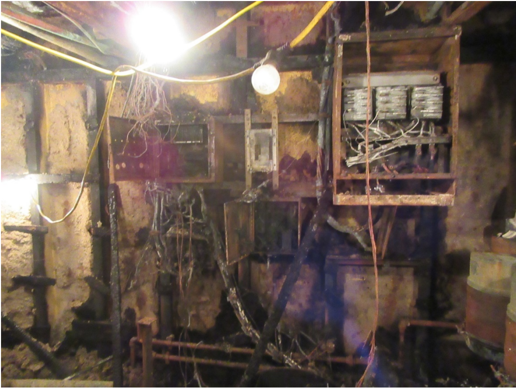
Generator Space Damage
