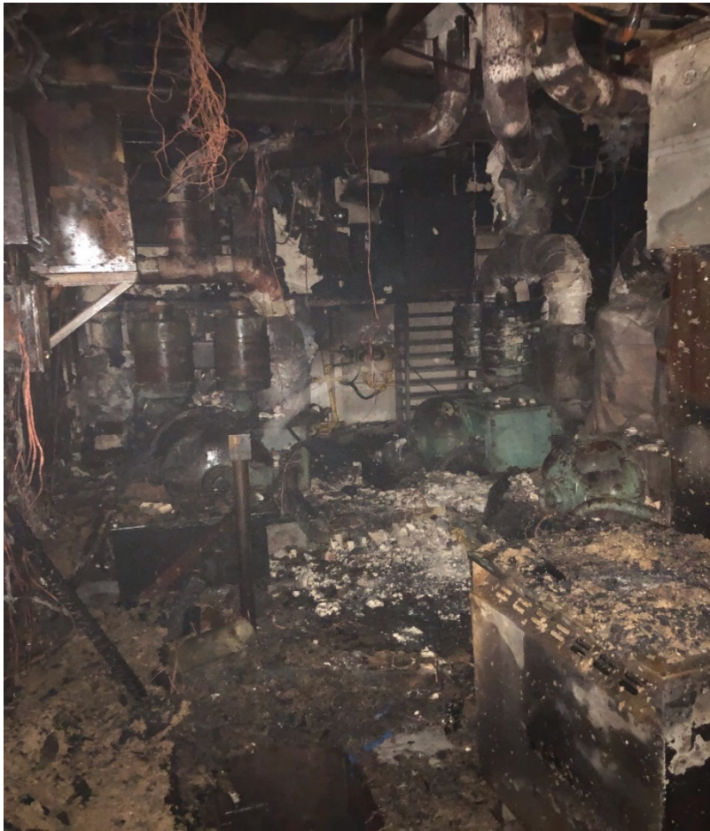
Generator Space showing the three generators
