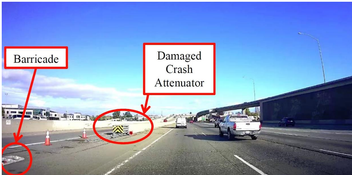
Figure 15. Southbound US-101 view depicting the precrash damaged condition of the crash attenuator, orange traffic cones, and a displaced Type 1 sawhorse-style barricade on March 22, 2018. (Source: CHP photo provided by passerby)
