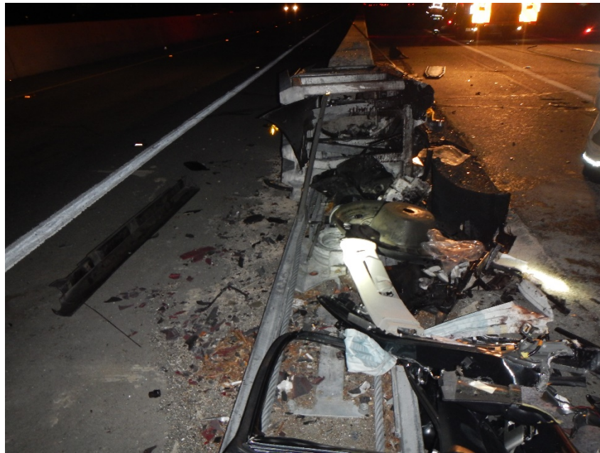
Figure 5 – Postcrash photo of crash cushion on November 14, 2015, at the exit ramp transition to SR-85.
