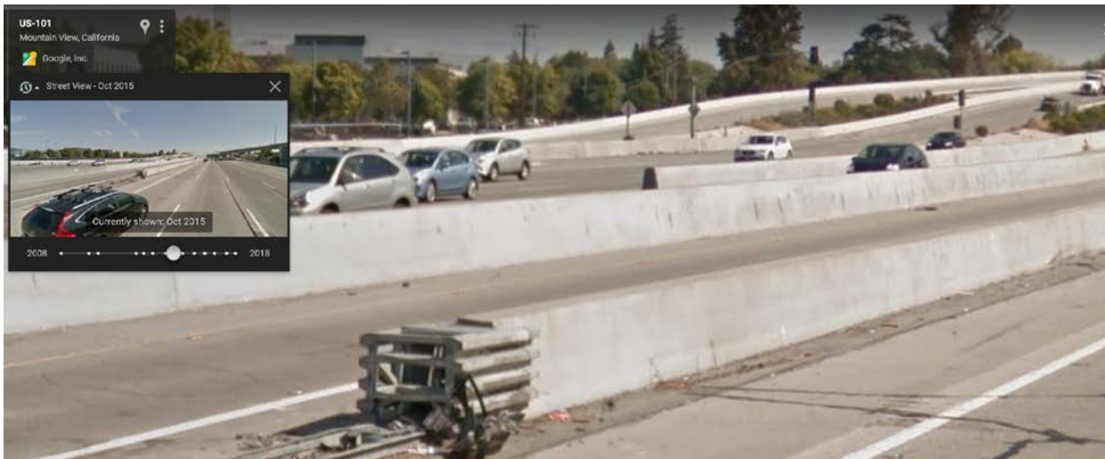
Figure 1 – Google Maps Street View image from October 2015 showing the crash cushion fully collapsed and missing the retroreflective object marker. This was the condition of the crash attenuator when the fatal traffic collision occurred on November 14, 2015.
