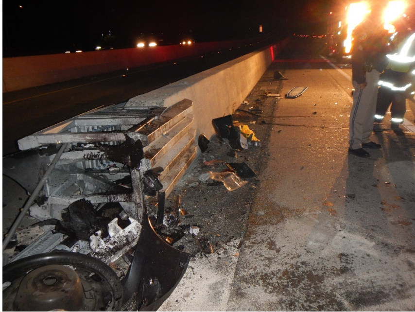
Figure 4 – Postcrash photo of crash cushion on November 14, 2015, at the exit ramp transition to SR-85.
