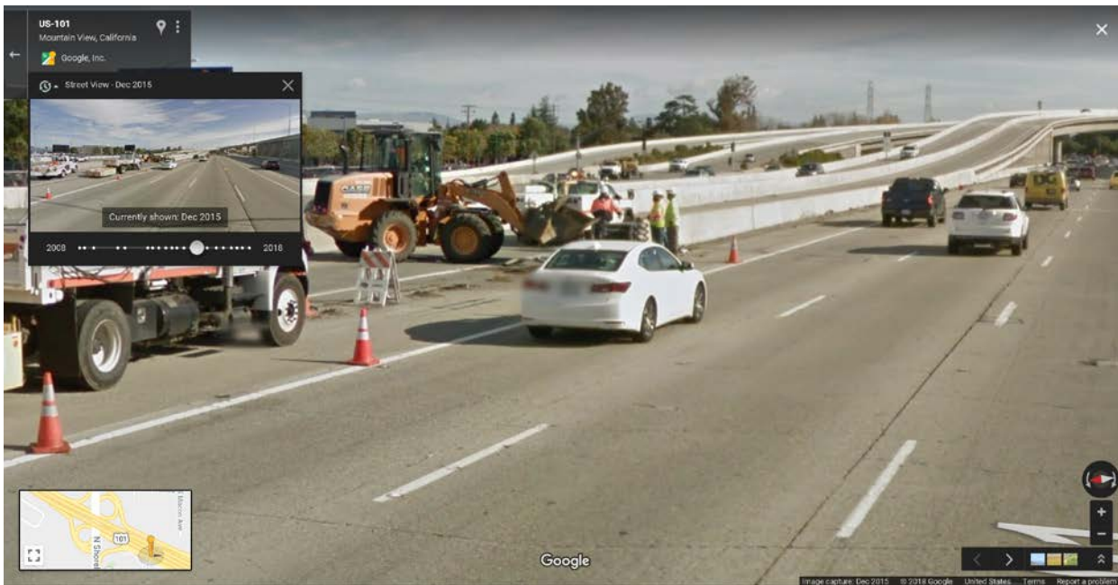
Figure 7F – Google Maps Street View image captured on December 23, 2015 showing the crash cushion being repaired by Caltrans.
