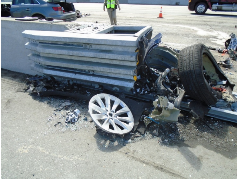
Figure 6C – Postcrash picture of damaged crash attenuator with Tesla vehicle components lodged inside of the hollow interior section of the crash cushion.
