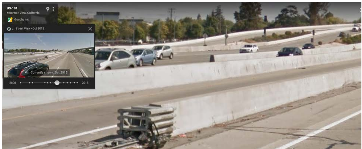
Figure 7D – Google Maps Street View image captured in October 2015 showing the crash cushion fully collapsed and missing the retroreflective object marker.
