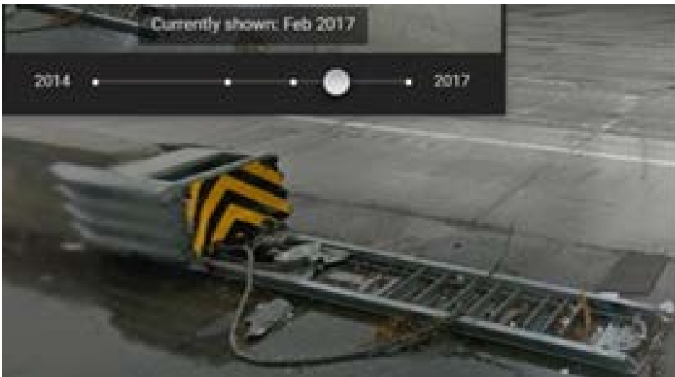
Figure 7K – Google Maps Street View image captured in February 2017 showing the crash cushion fully collapsed and the broken wire cable.
