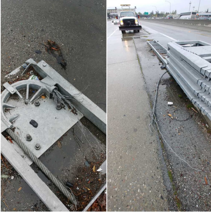
Figures 7G and 7H – Photos taken on March 20, 2018 by a Caltrans worker depicting the damage to the crash attenuator and wire cable.
