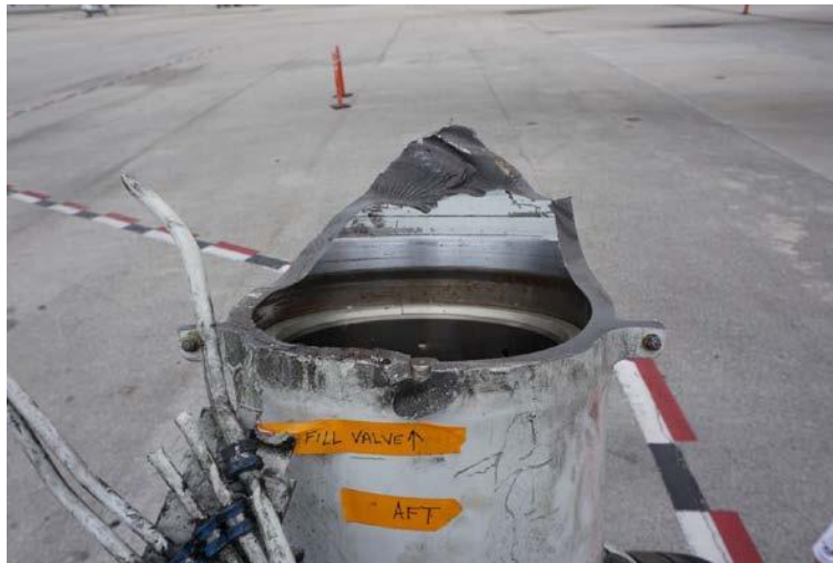
Aft Side of Lower Section of Left Main Landing Gear Cylinder and Air Fill Valve Bore
