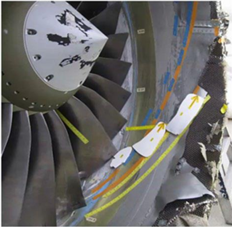
Figure 6 – Possible Fan Blade Fragment Forward Helical Trajectory from Fan Case to Inlet
