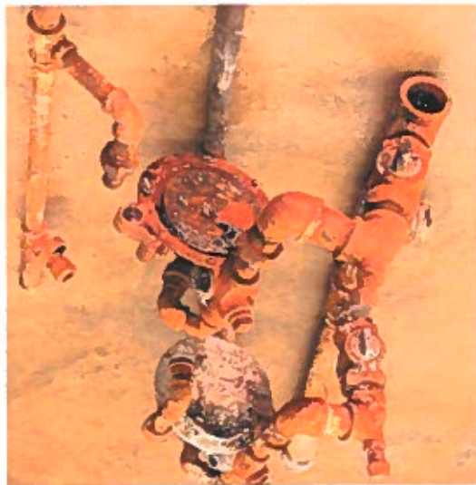
Deflection of Vent Piping
