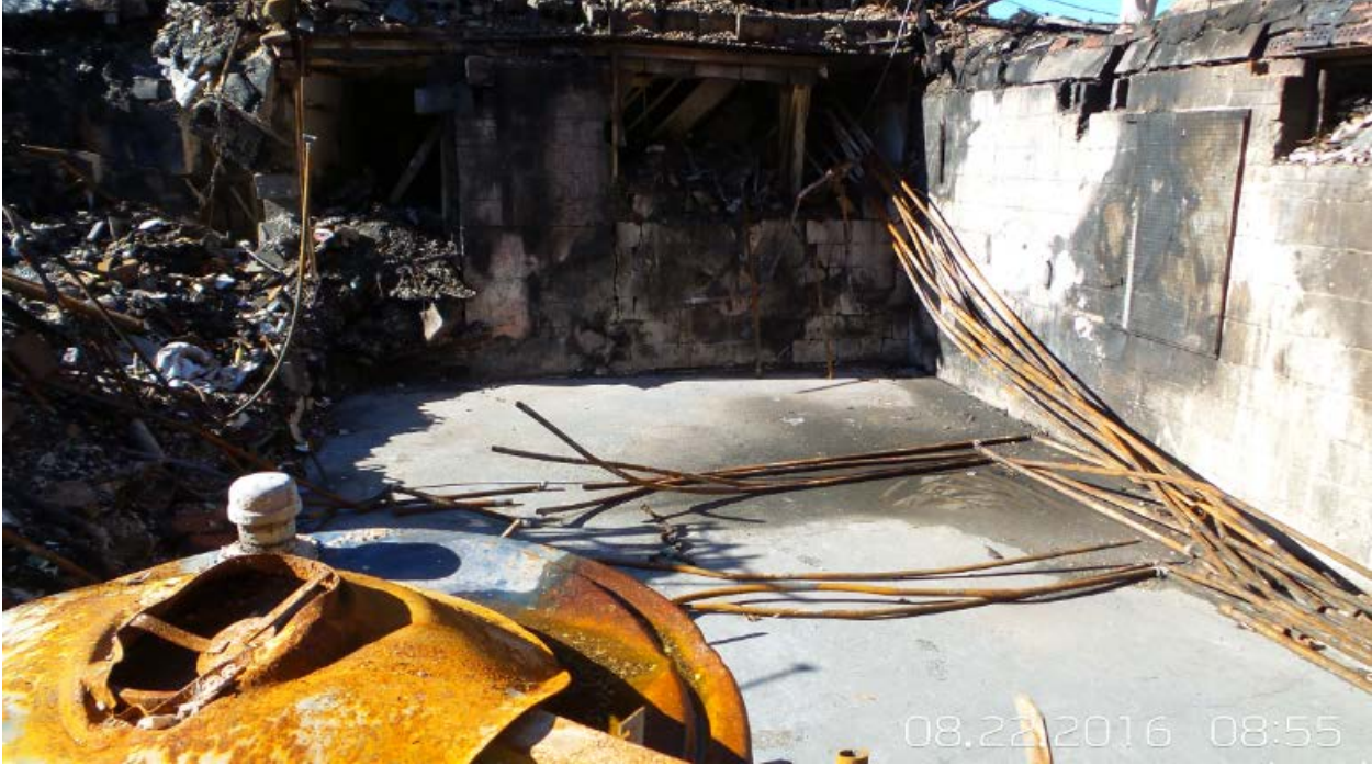
Appendix B: Photo coverage of the basement perimeter and accident area at 8701 Arliss Street by Kay Management representative.
