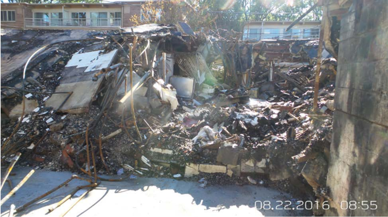
Appendix B: Photo coverage of the basement perimeter and accident area at 8701 Arliss Street by Kay Management representative.
