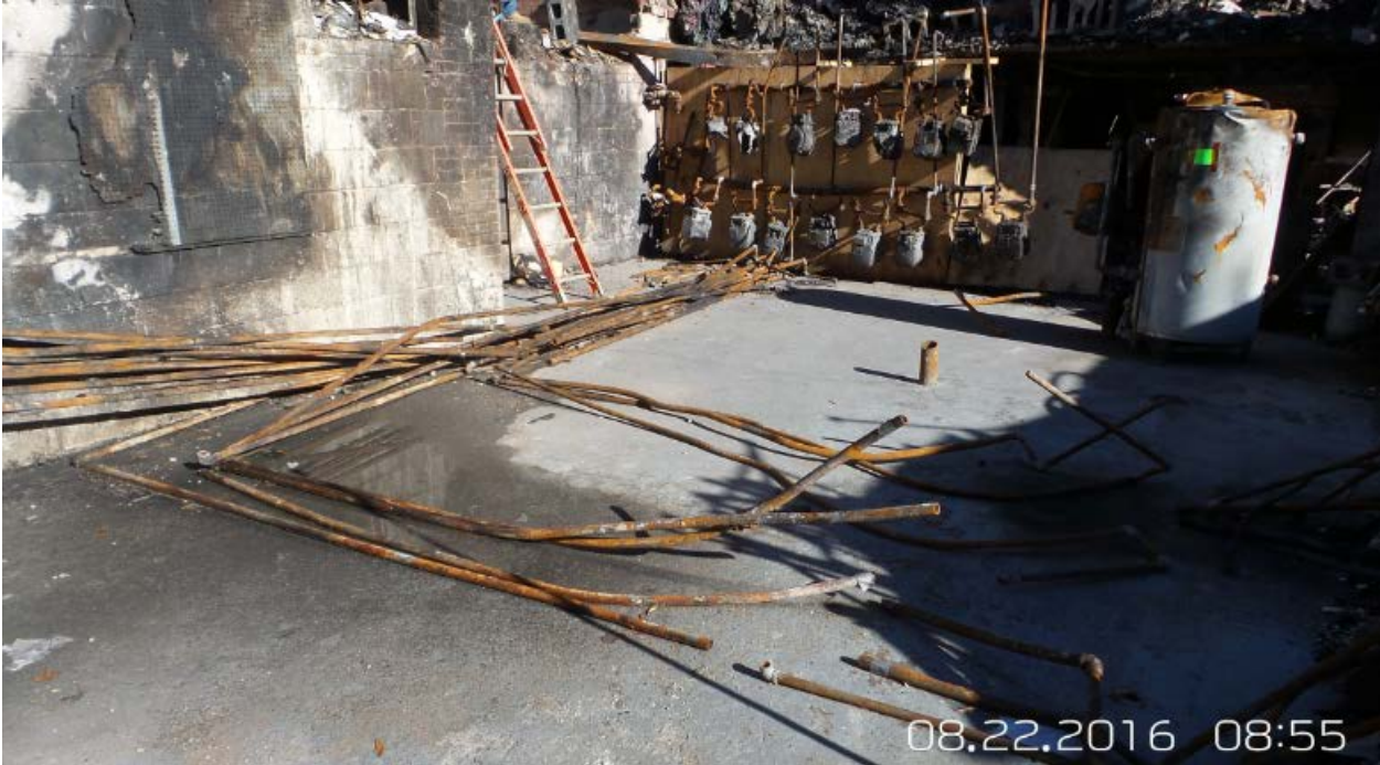
Appendix B: Photo coverage of the basement perimeter and accident area at 8701 Arliss Street by Kay Management representative.
