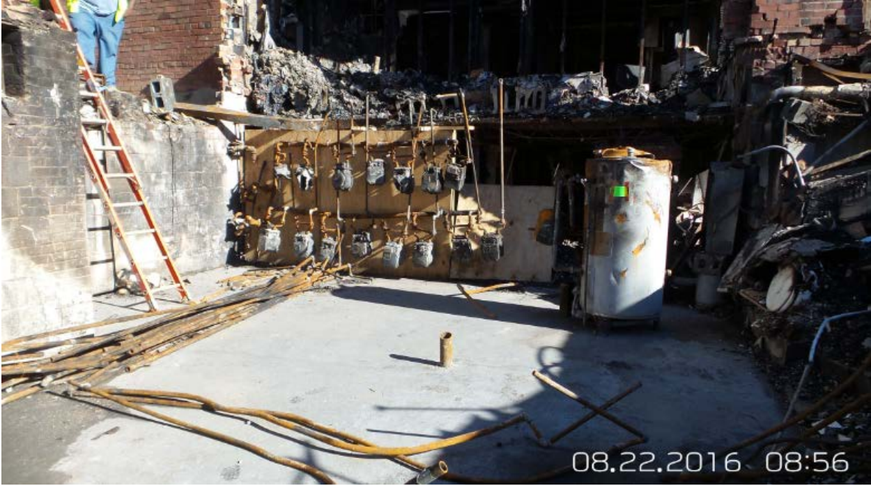
Appendix B: Photo coverage of the basement perimeter and accident area at 8701 Arliss Street by Kay Management representative.
