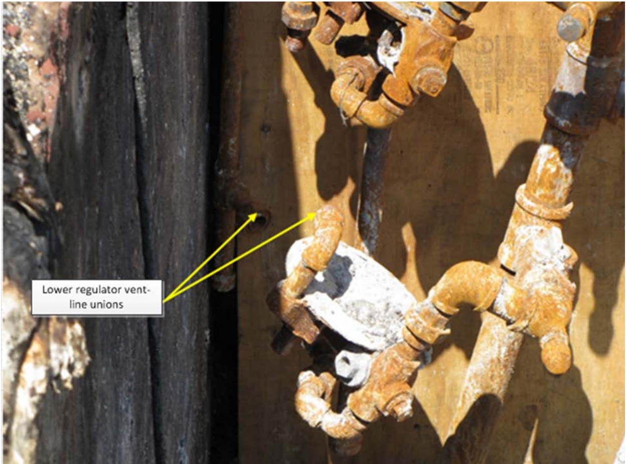
Figure 9: Damaged lower service regulator disconnected from the vent pipe at the union, and connected to the inlet service pipe and outlet service pipe.
