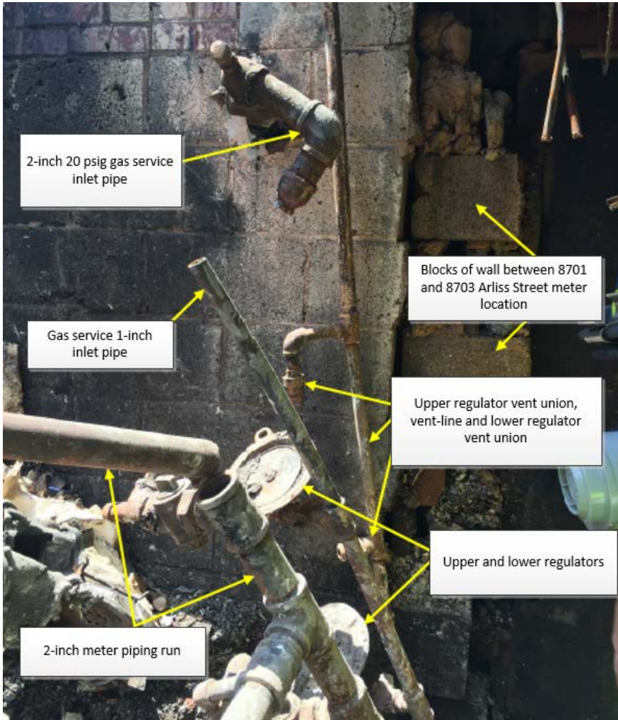
Figure 5: The meter and piping orientation before reconstruction by ATF. Source: WG
