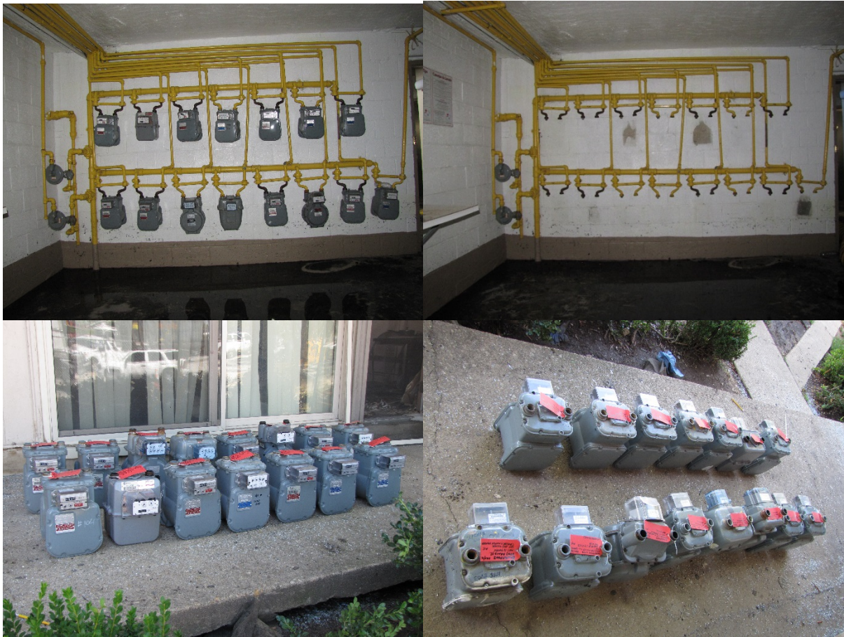
Figure 19: 8703 Arliss Street Silver Spring WG meter set piping, meters prior to and post removal.
