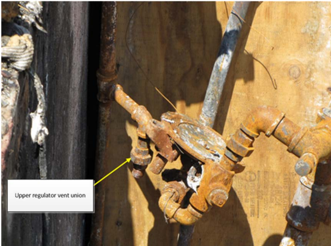
Figure 8: Damaged upper service regulator found broken from the vent pipe, and connected to the gas inlet service pipe and outlet service pipe.
