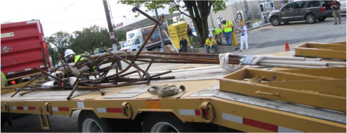
Figure 17: 8701 Arliss Street Silver Spring, Apartment Customers Gas Piping on Trailer bed.
