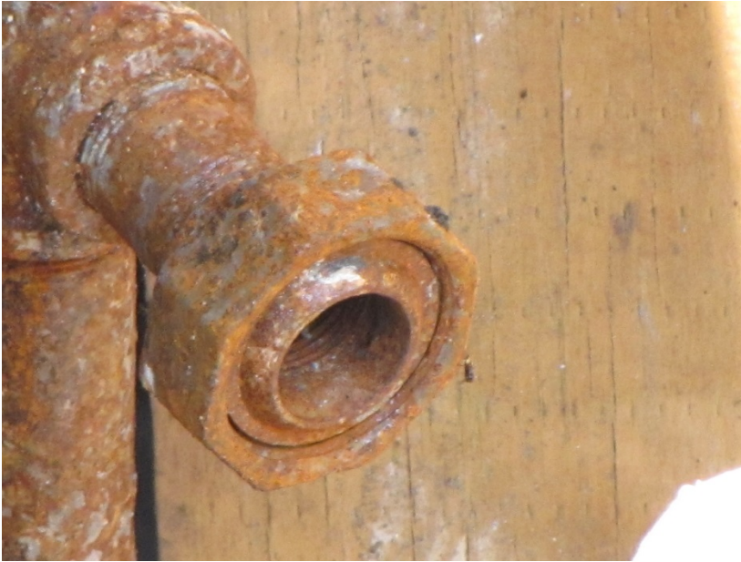
Figure 10: Female connection to the 1-inch vent pipe and the second damaged lower service regulator at 8701 Arliss Street.
