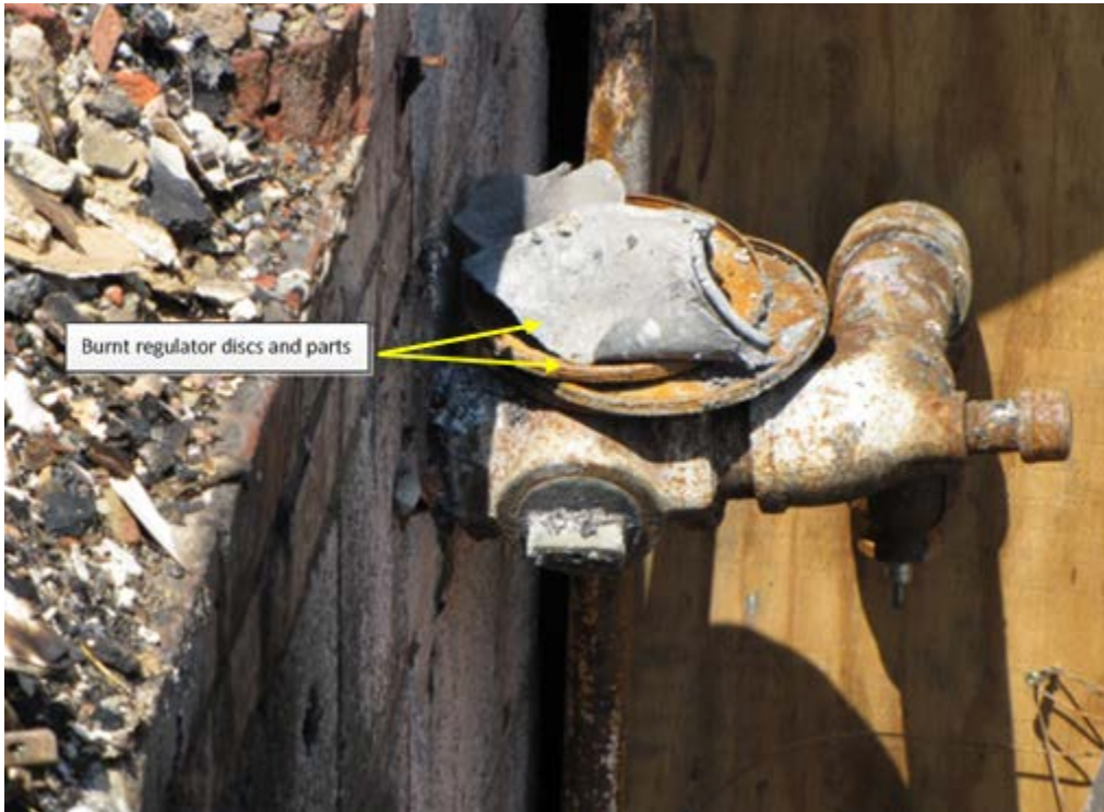
Figure 7: The 2-inch gas service entrant pipe, service valve, 2-inch reducing tee with capped 3/4-inch elbow, 2-inch downward facing elbow with plugged 1-inch service pipe connection.
