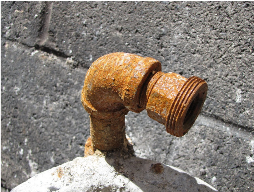
Figure 11: Male union connection to the 1-inch vent pipe and the second damaged lower service regulator at 8701 Arliss Street.
