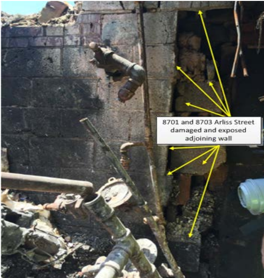
Figure 4: Gas meter piping, appurtenance and damaged adjoining wall to 8701 and 8703 Arliss Street following the explosion. Sources: WG
