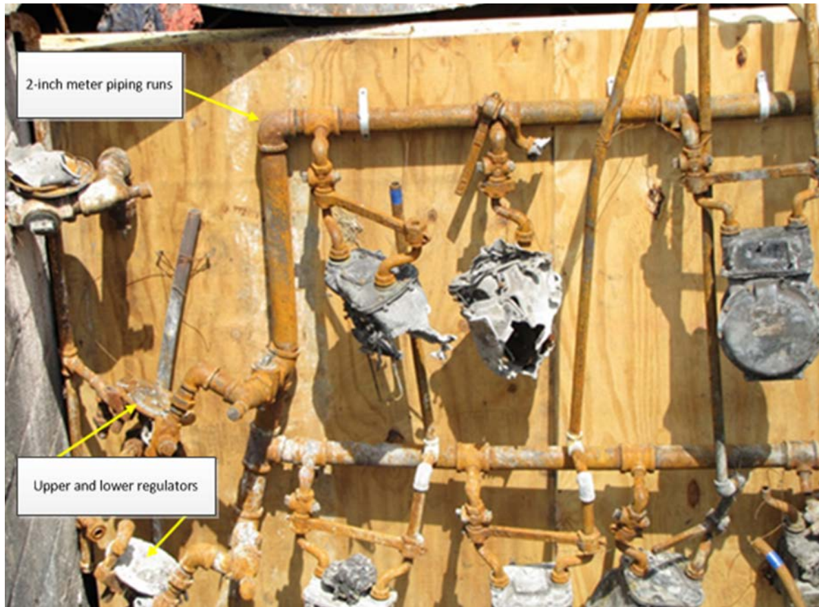
Figure 6: Close up view of two service regulators and the two 2-inch piping runs connected to customer meters.
