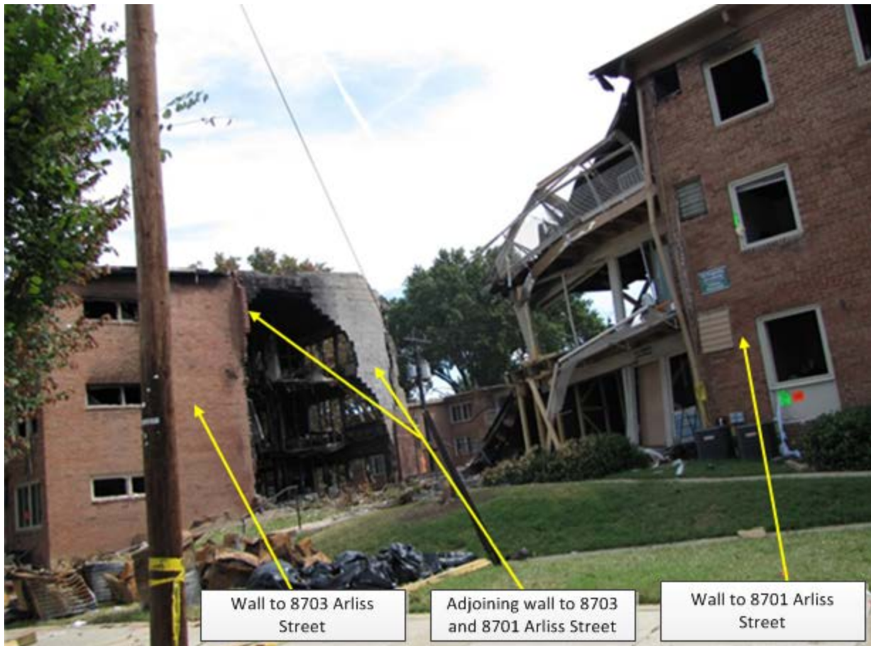
Figure 1: shows the standing remnants of 8701 Arliss Street (to the right) and the adjoining 8703 Arliss Street on the left.
