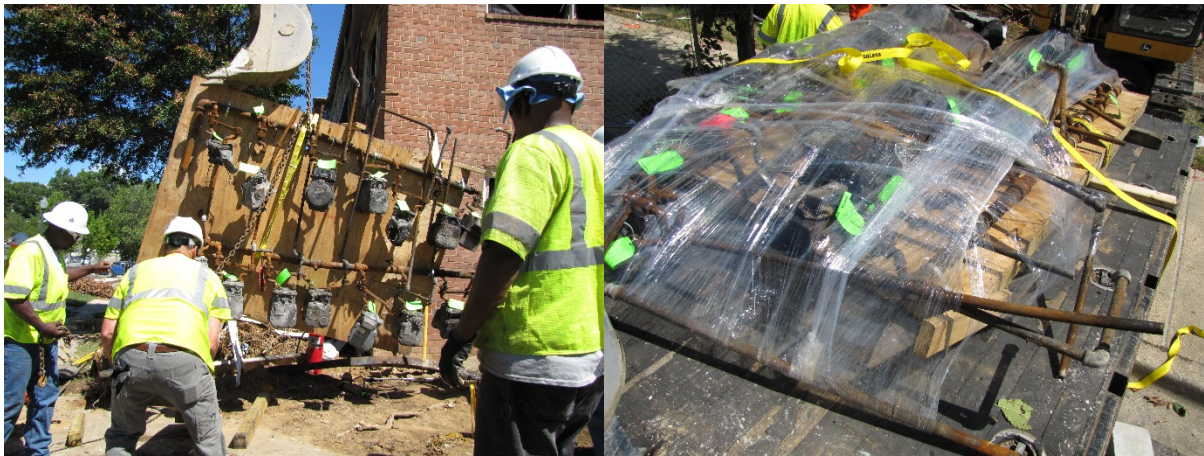
Figure 16: Reassembled meter rack containing 15 damaged customer meters and piping from 8701 Arliss Street, Silver Spring, MD.
