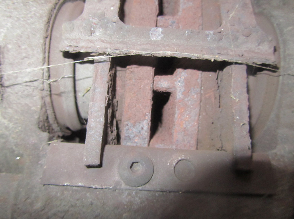
Vehicle Photo 12 – 2003 Blue Bird School Bus, Left Rear Brake Showing Missing Lining
