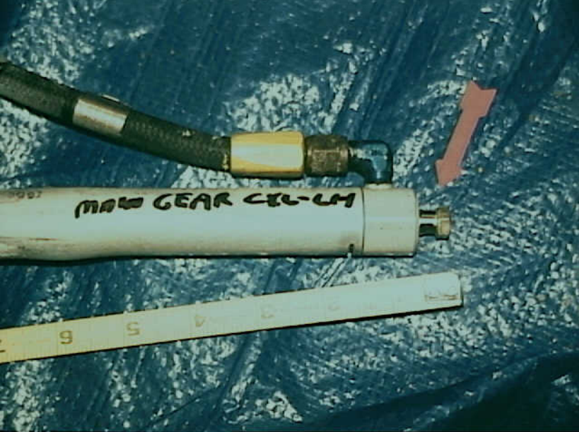
Airworthiness - Photo 18. Close-up view of the exposed portion of the stabilator trim jackscrew. (NTSB-T18)
