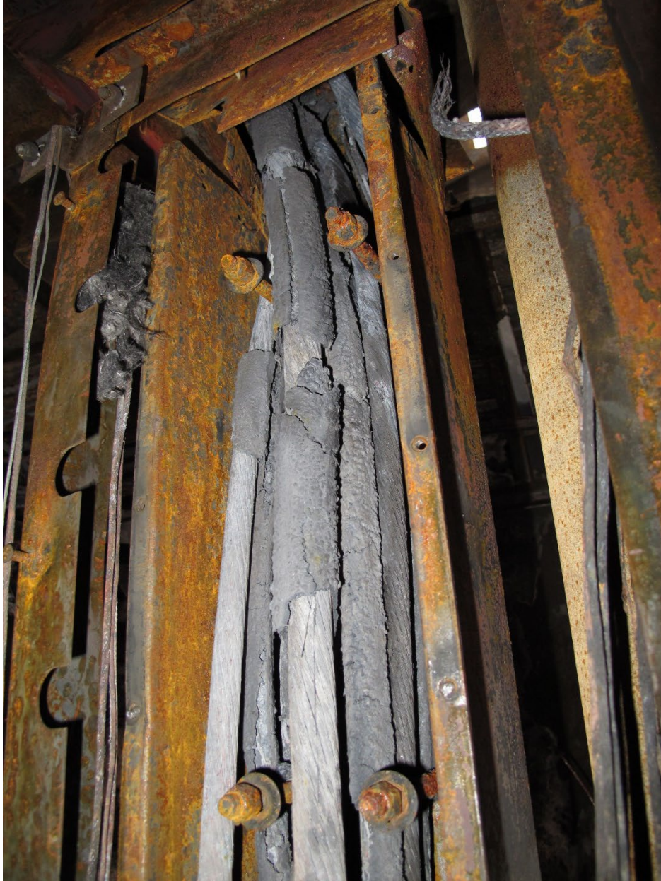
Figure 15. Electrical cabling found within power cable cabinet shown in Figure 14. (NTSB)
