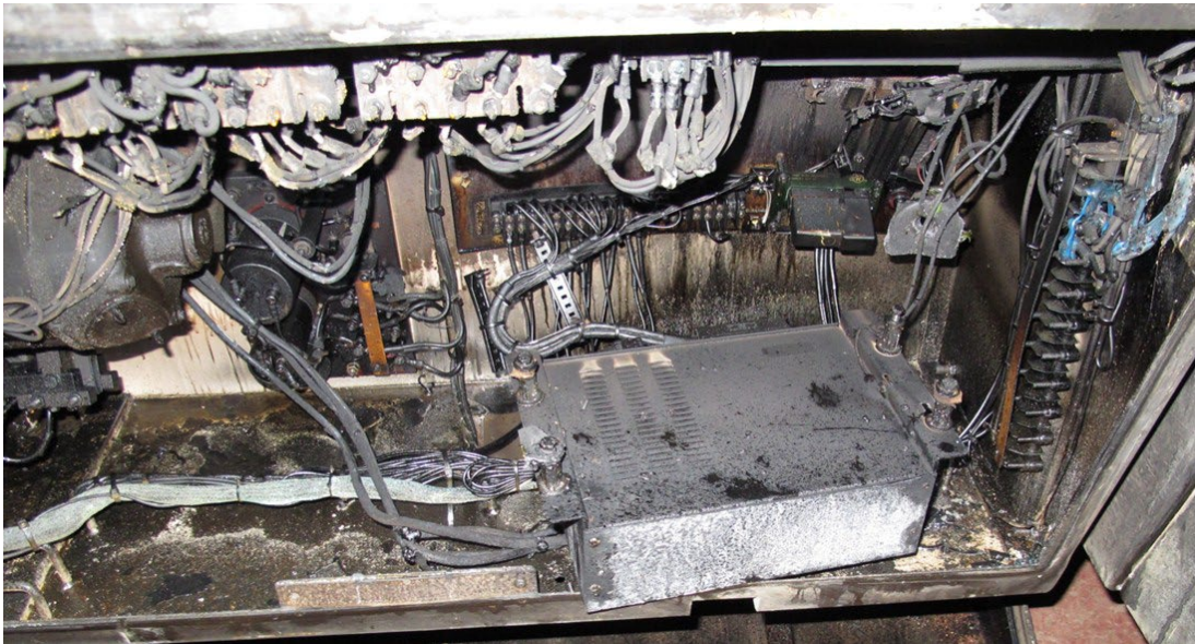
Figure 10. Thermal damage to adjacent control equipment. (NTSB)
