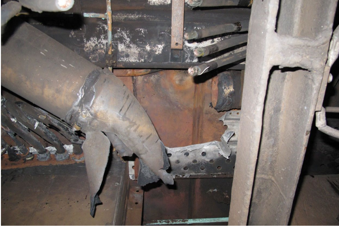
Figure 21. Thermal damage to polymeric and aluminum components found in the undercarriage approximately centerline. (NTSB)
