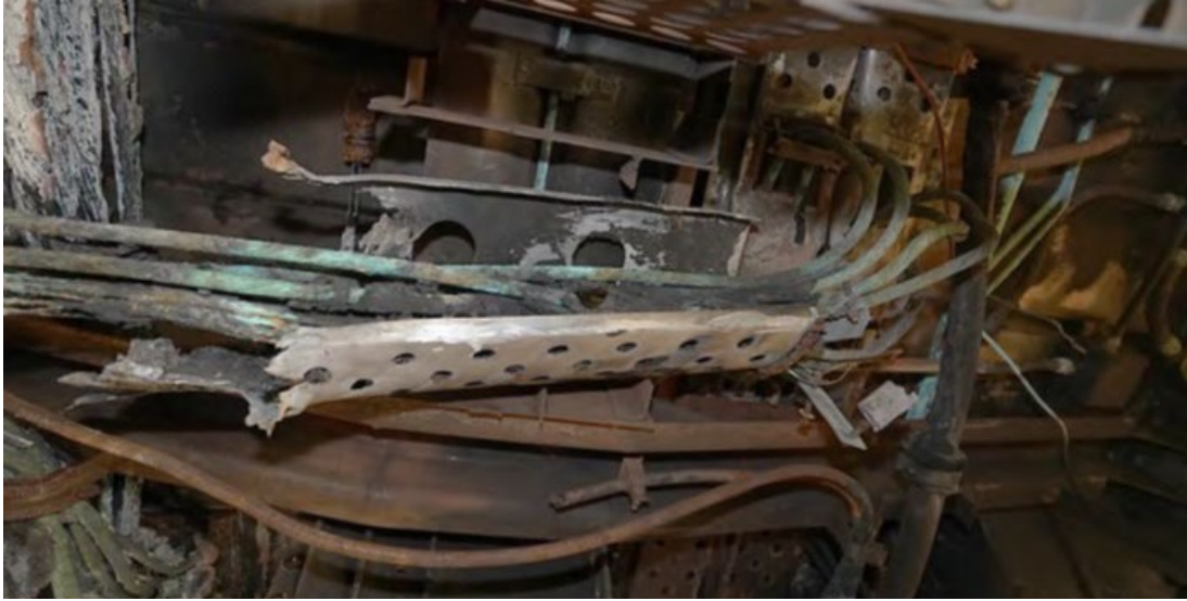
Figure 7. Thermal damage to aluminum cable trays. (SEPTA)
