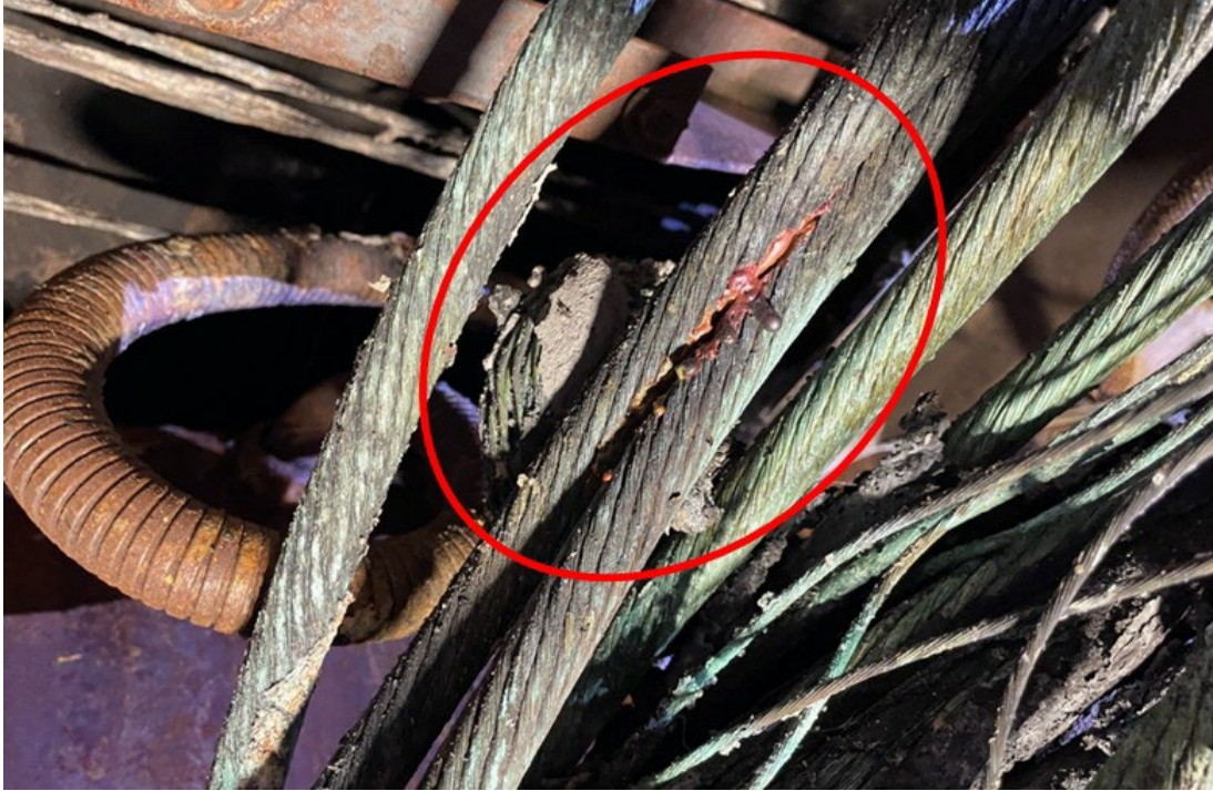
Figure 9. Arcing damage (circled in red) on the 31MD (motor #1 field winding) and 31MA (motor #1 armature winding) wires, found in an area aft of the intake to the double-end blower on the left side of the car. (NTSB)
