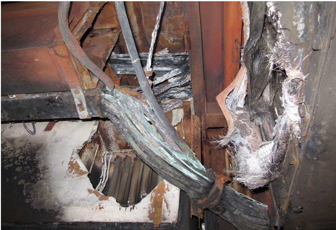
Figure 22. Section of thermal damage to wiring underneath Car 114.
