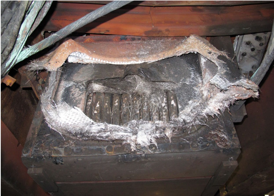
Figure 23. Damage to smoothing reactor cooling coil insulation. (NTSB)
