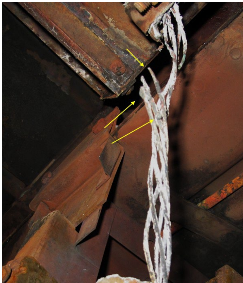
Figure 8. Beading (indicated by yellow arrows) on electrical conductor ends found on the left side of the undercarriage. (NTSB)
