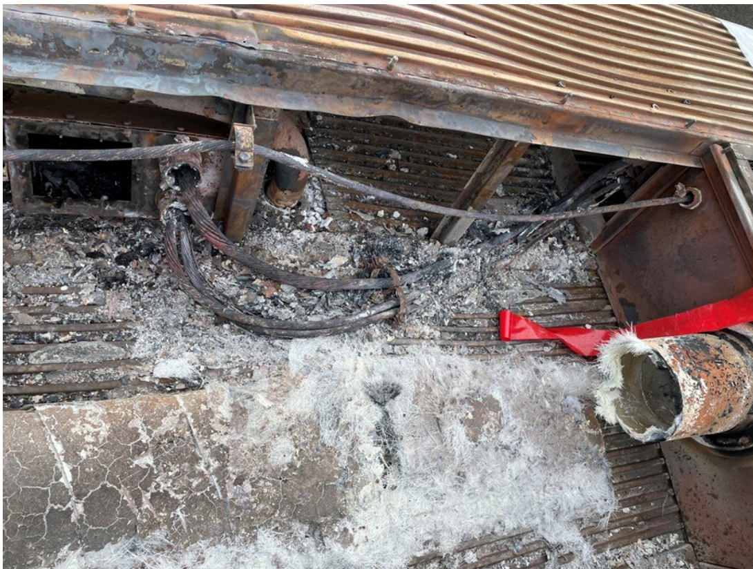
Figure 11. Damage to ducting and wiring found on the roof of Car 132. (FRA)
