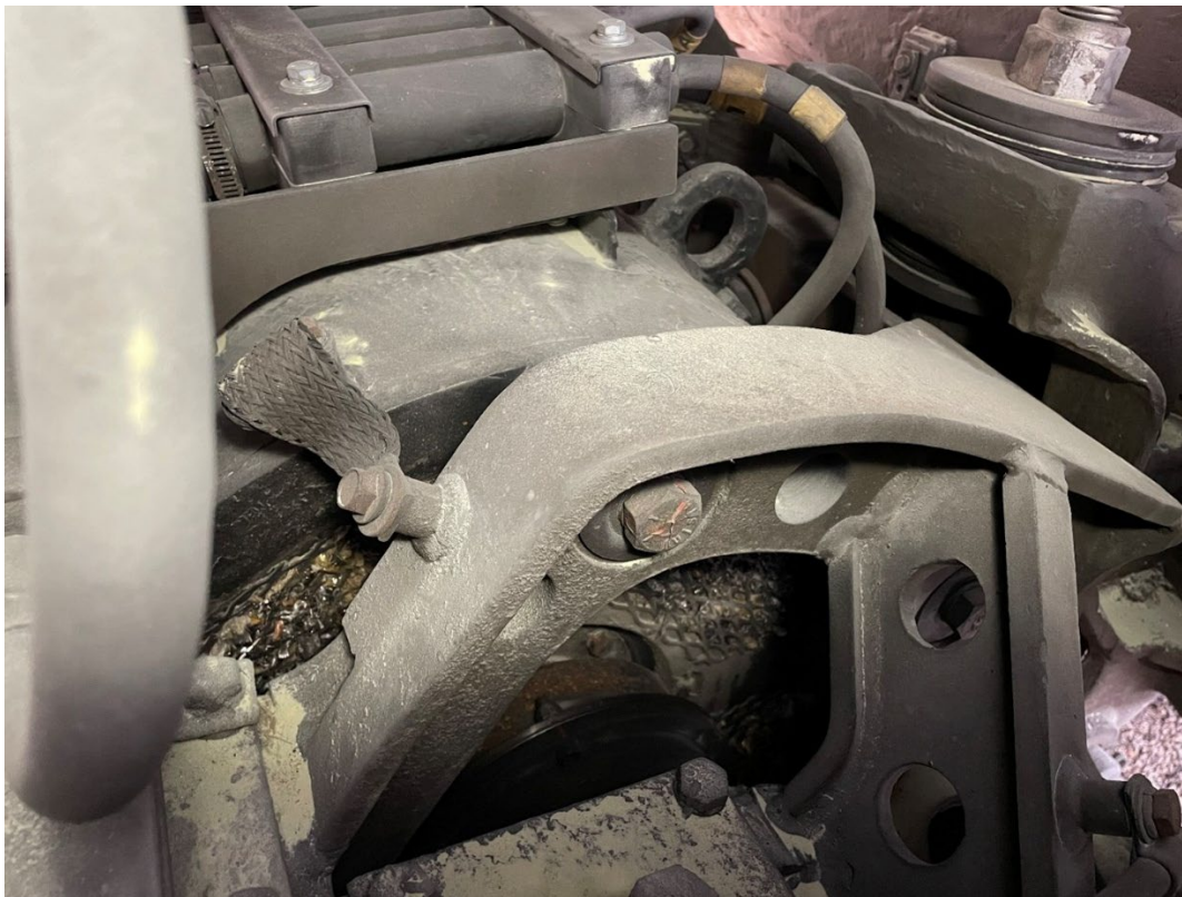
Figure 9: SEPTA Car 396 Traction Motor Close-up
