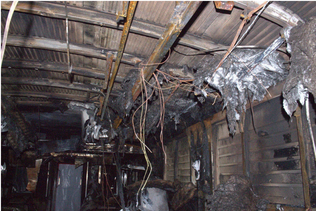
Photo 2 Photograph of the damage to the interior of the Silver Liner IV Car 132 showing the extensive damage to the ceiling and sidewall of the rail car. (Source: NTSB)
