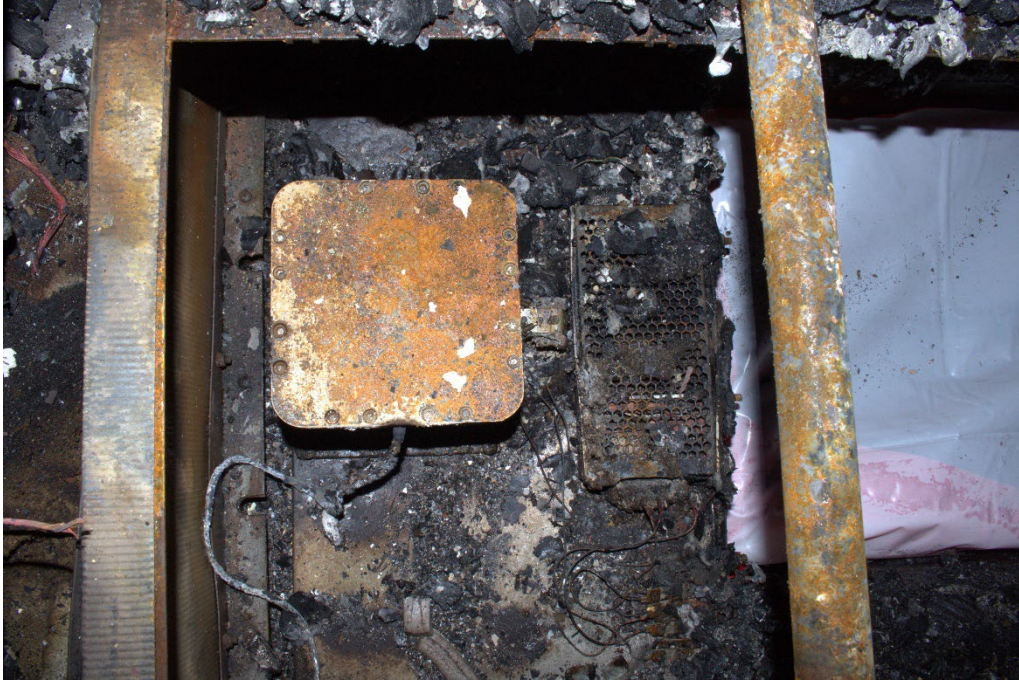
Photo 9 A closeup of one of the electronic modules still bolted to the frame in Car 132 prior to removal by investigators. (Source: NTSB)
