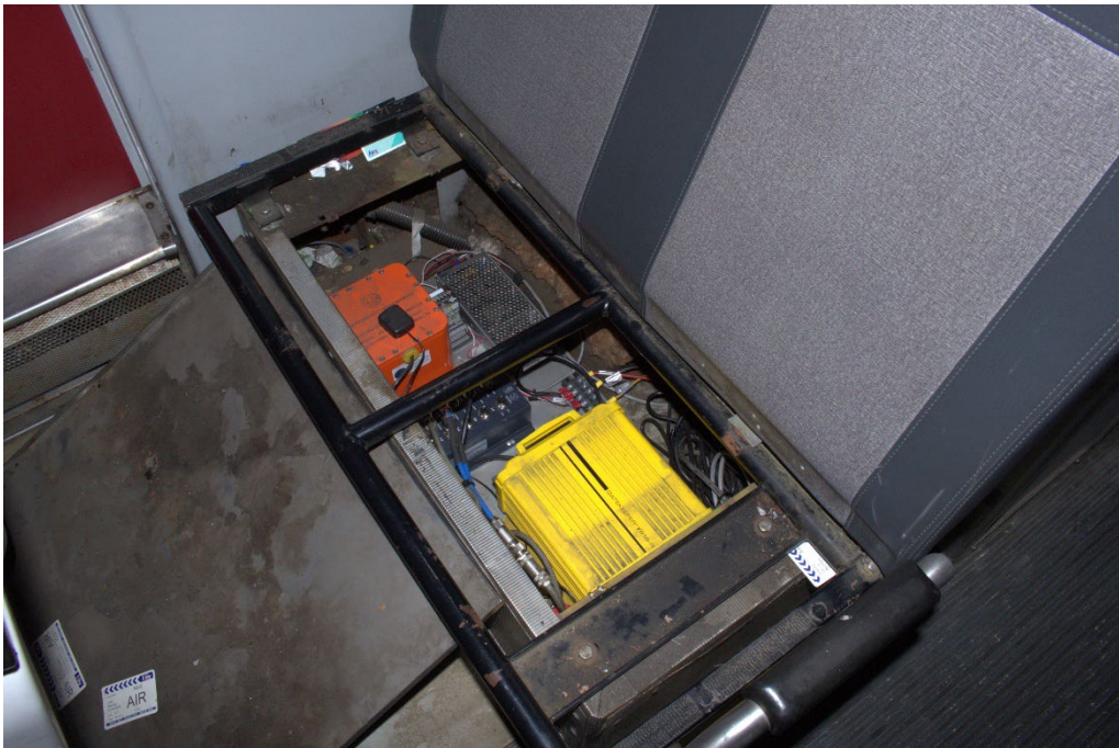
Photo 8 Image of the electronic recorder modules, seen here in Car 131, that are located underneath the mid-car seat in each of the rail cars. (Source: NTSB)
