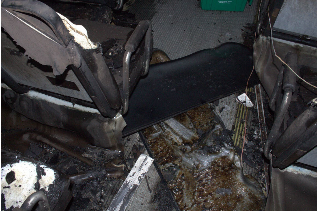
Photo 5 Closeup of the damage to one of the rail car windows caused by the intense heat. (Source: NTSB)
