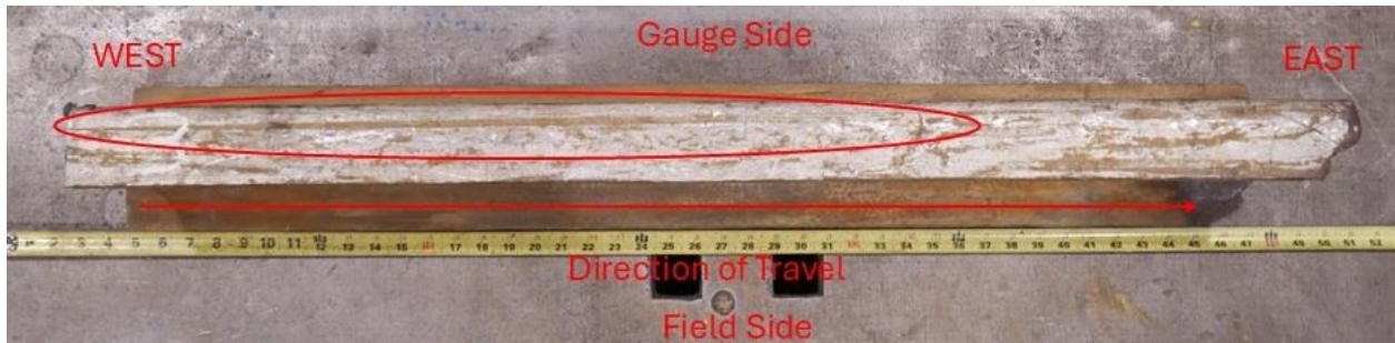
Image 4: A composite image of the railhead showing the batter with the damage caused by wheel ride circled in red.
