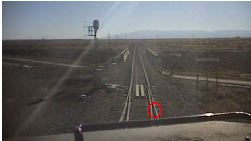
Figure 3 – Photo from the outward facing camera of lead locomotive (BNSF 9015) showing a broken rail on the north rail of Main Track No.1 at MP 109.654 (Photo courtesy of NTSB Operations Group Factual Report)
