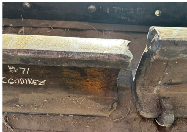
Figure 4 – Photo showing the break in the thermite weld at MP 109.654 (Photo courtesy of NTSB)
