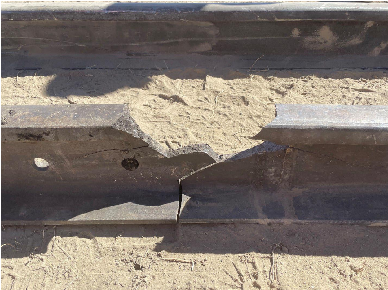
Figure 2. Photograph of breakout in the rail located 71” north of the initial broken rail (weld #71). This rail broke under the last train prior to the derailment as confirmed in video footage.
