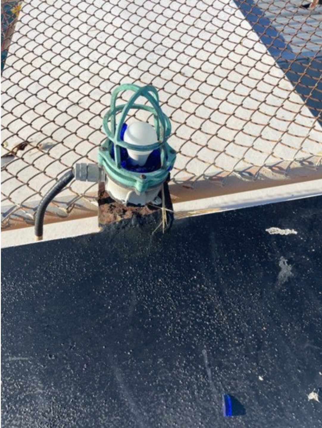
Figure 12. Photo of the northwest elevation, center light, immediately after the accident. Photo courtesy of Walter Oil and Gas.
