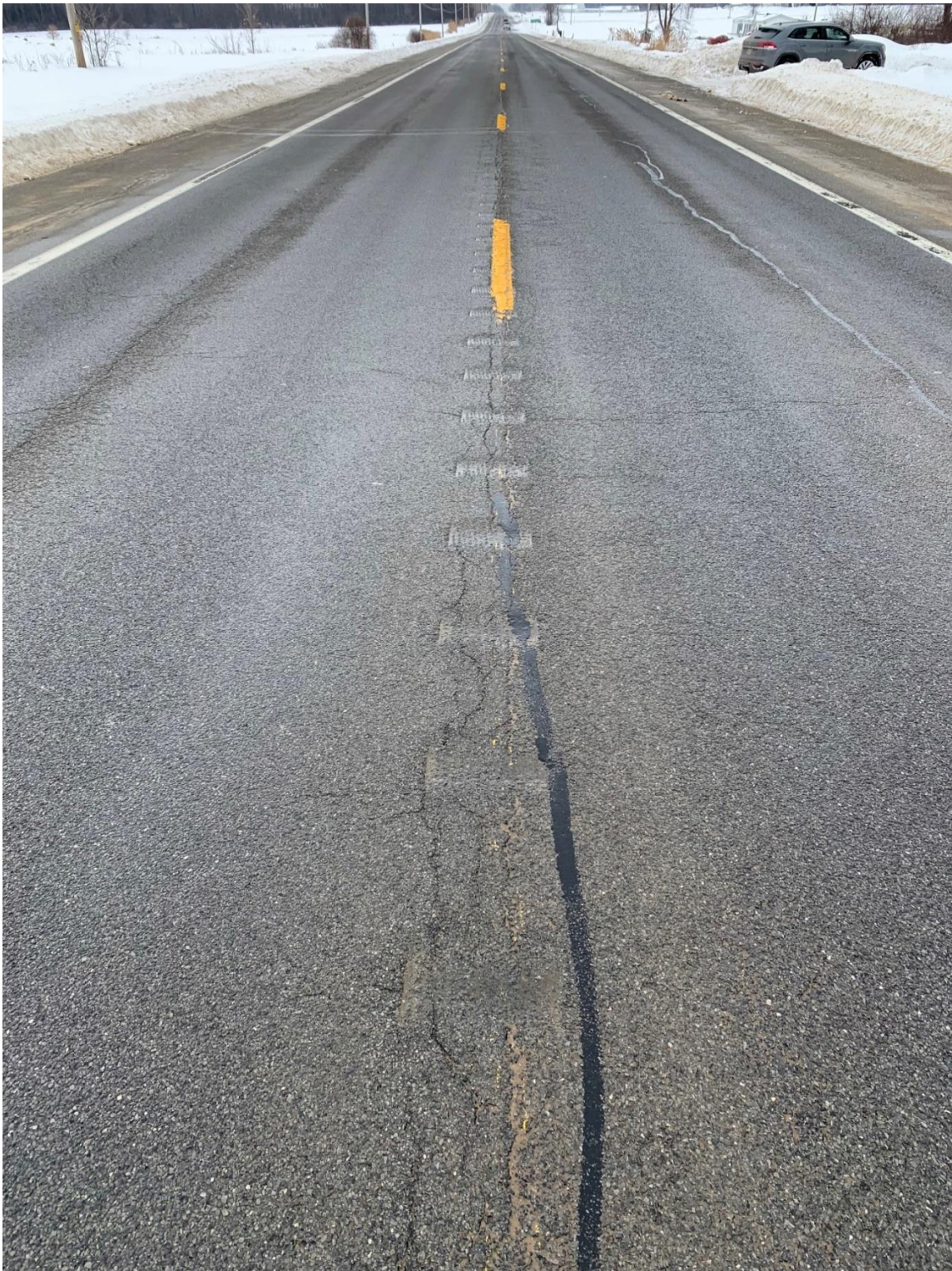
Highway Factors Photograph 1 – View of centerline rumble strips along State Route 37 in the vicinity of the crash
