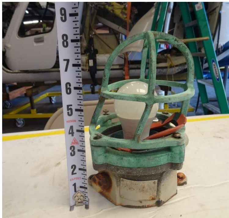
Figure 10. The damaged blue-colored light.
