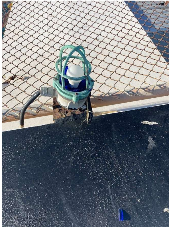
Figure 9. The damaged blue-colored light found at the helipad. The platform operator stated they had cut the light housing's installation bolts to facilitate its removal from the helipad. (Image courtesy of Walter Oil)
