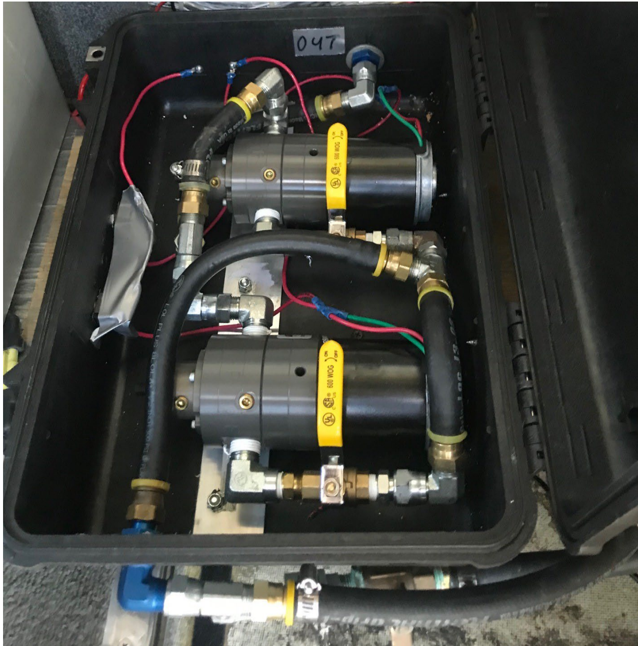
Figure 6. Photo of transfer pump installation. (Courtesy of Flight Contract Service)
