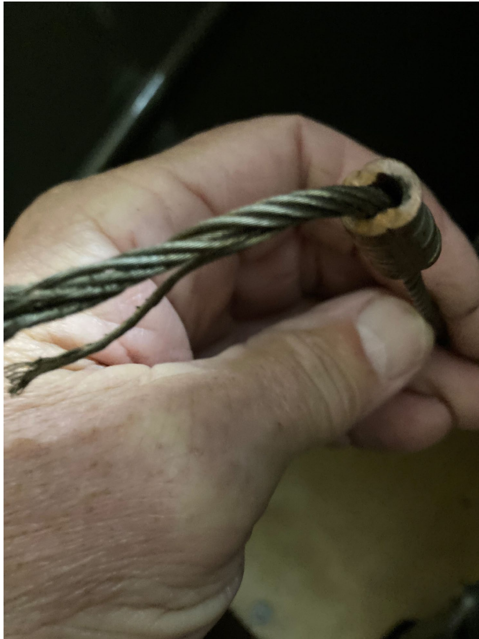
Photo 3 - View of the control cable and nicopress swage. Courtesy of the owner.
