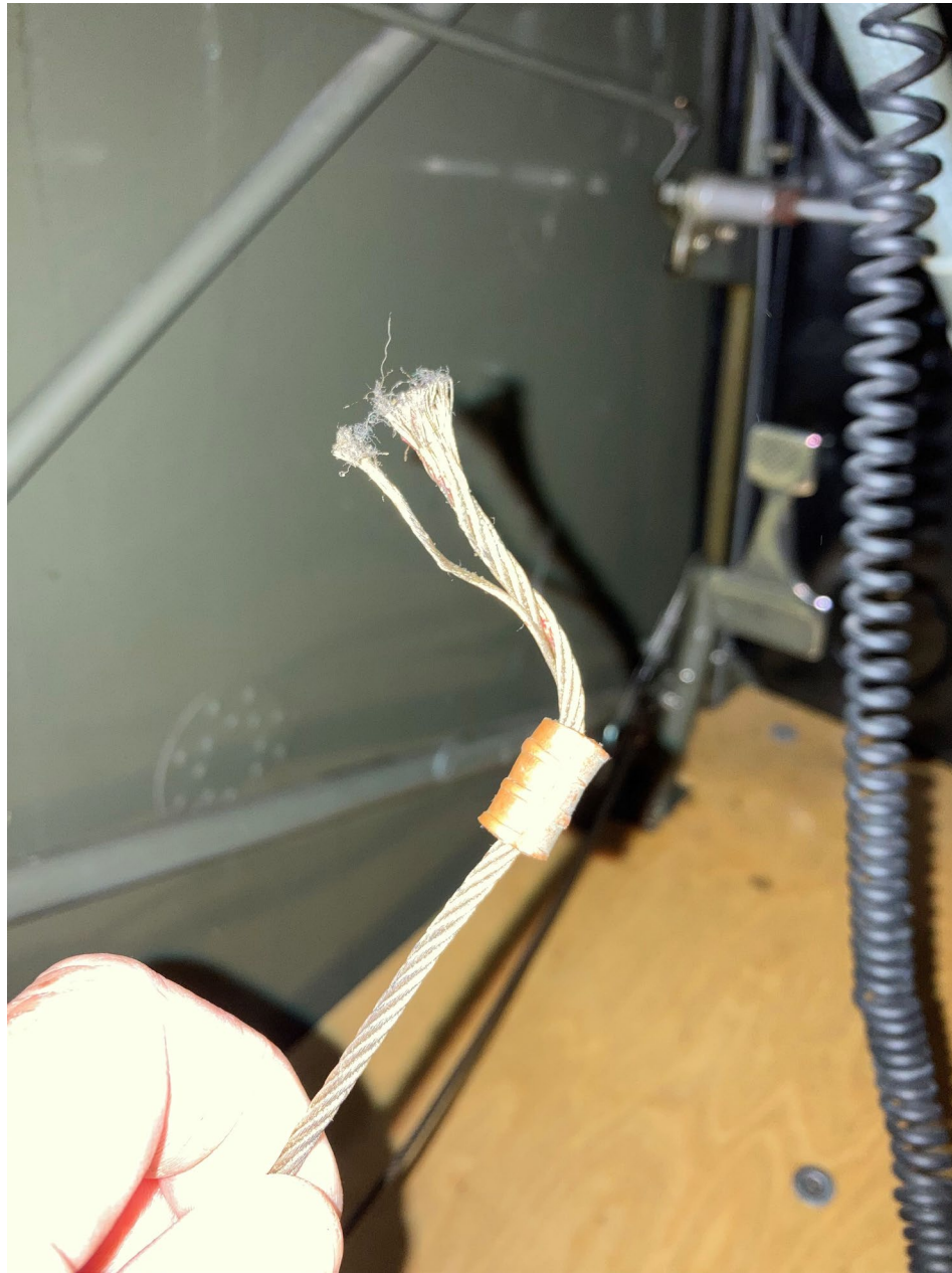
Photo 4 - View of the control cable and nicopress swage. Courtesy of the owner.
