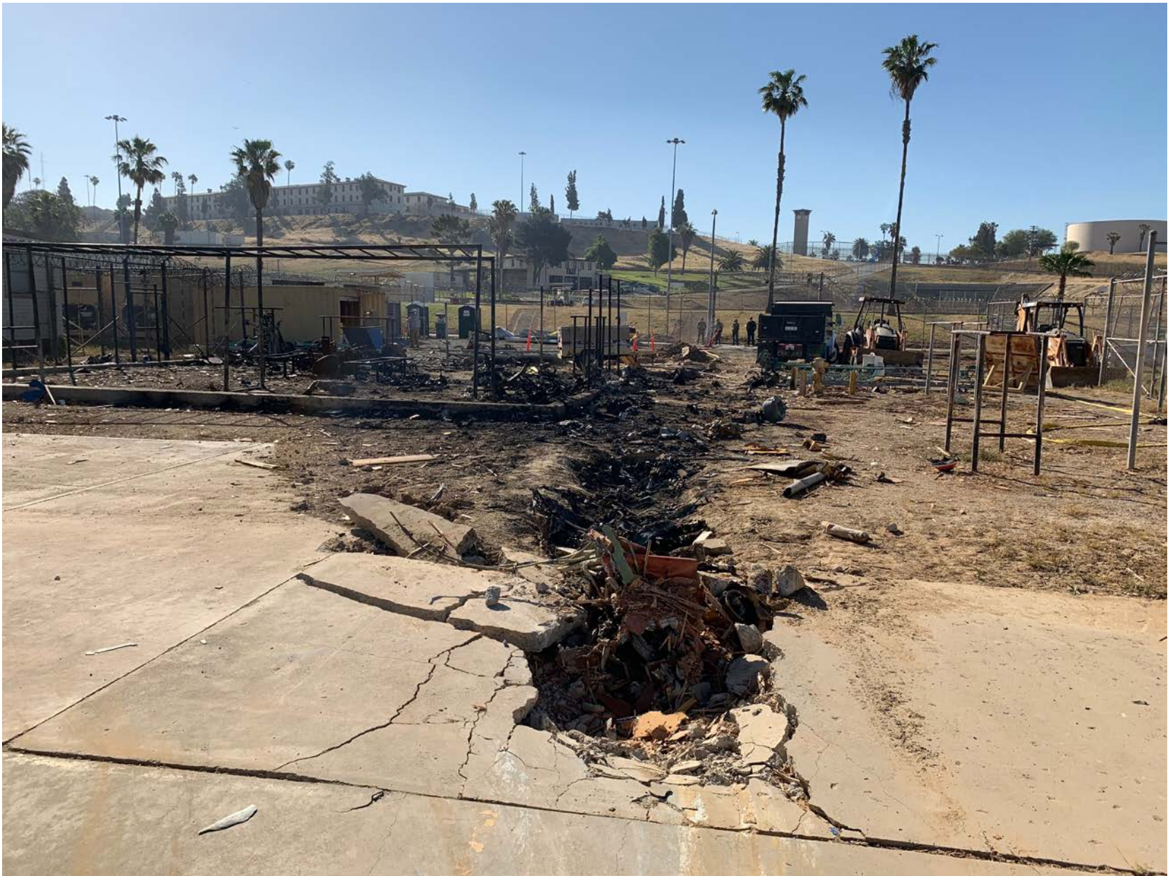
Photo 2 - View of the accident site.
