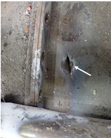
Figure 14. Exhaust duct penetration
