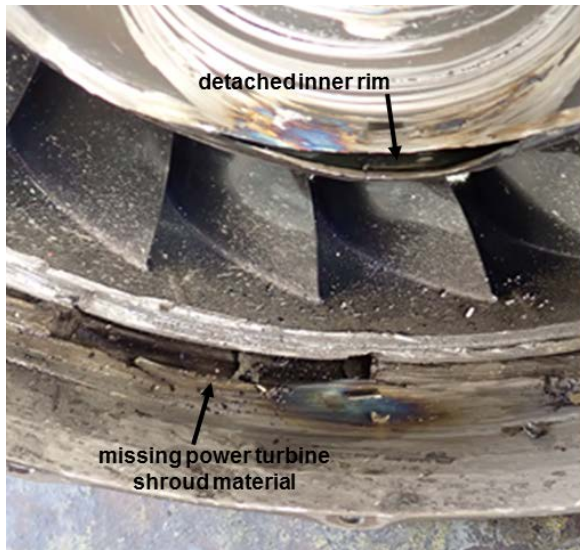
Figure 27. Detail, downstream power turbine vane ring and baffle assembly
