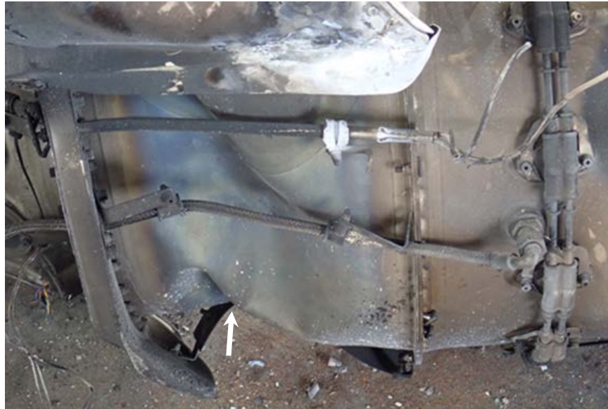
Figure 13. Exhaust duct distortion
