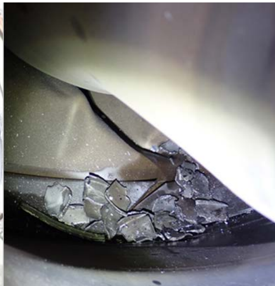
Figure 36. Airfoil debris lying in exhaust duct
