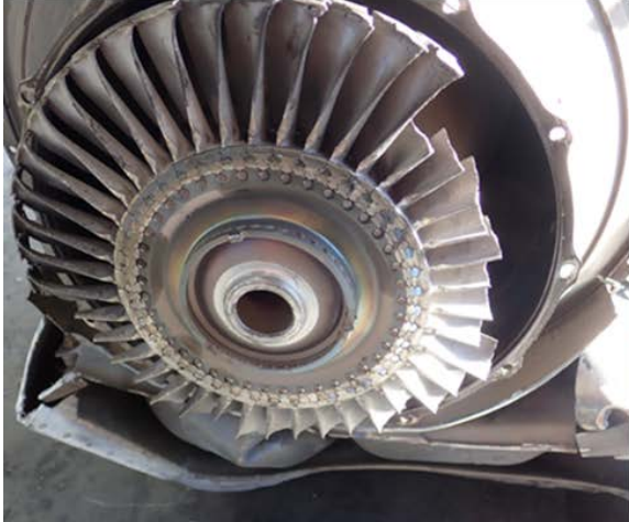
Figure 53. Power turbine with power turbine vane ring and baffle assembly removed
