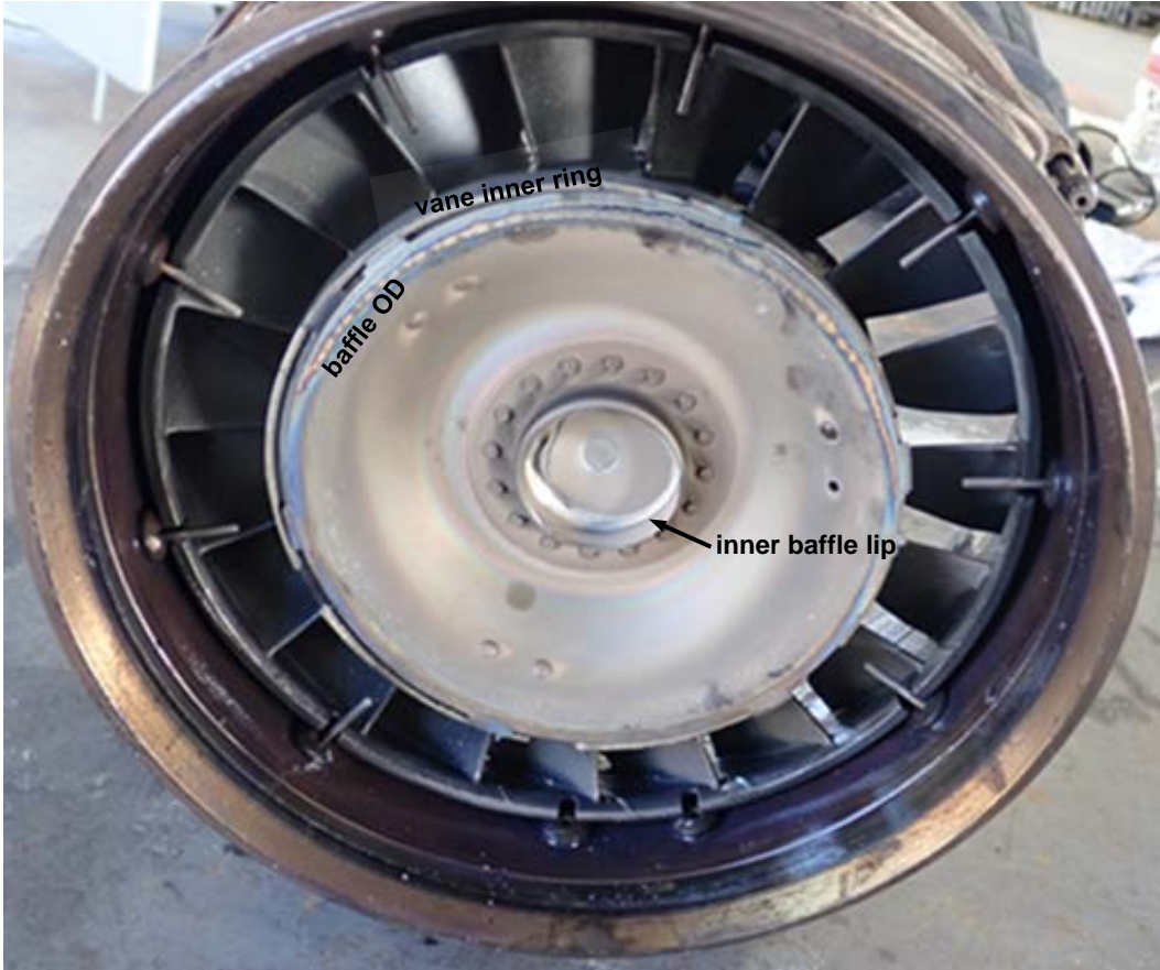
Figure 51. Upstream face of power turbine vane ring and baffle assembly showing rotational damage
