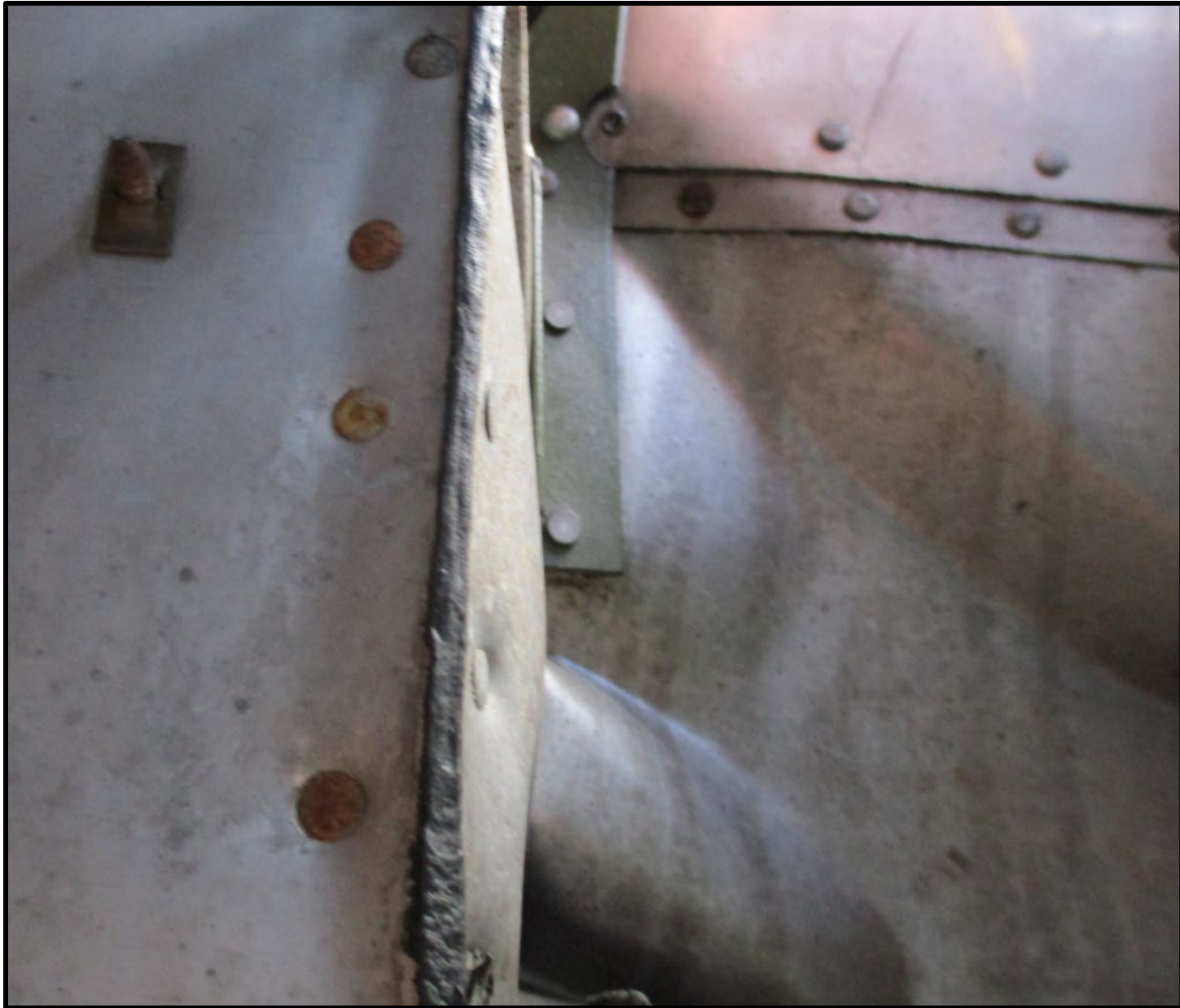
Figure 2: Wrinkled Firewall (photo provided by FAA)
