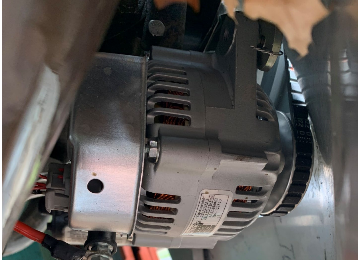
Figure 24. View of alternator attached to engine.
