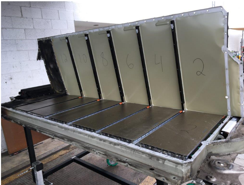
Burbank Inspection Photo 46: cover partially removed and bent upwards, left side modules numbered
