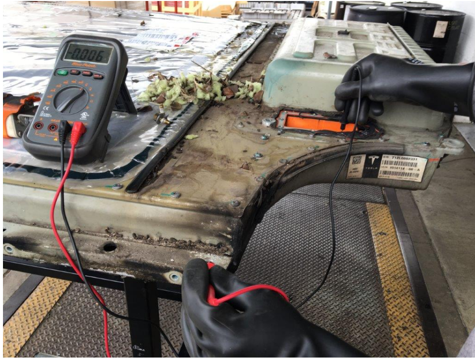
Burbank Inspection Photo 37: view showing voltage test to forward terminal of battery case
