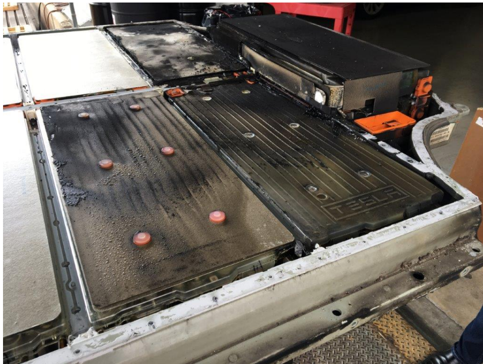
Burbank Inspection Photo 48: right front with covers removed and insulation layer of 13 and 15 removed
