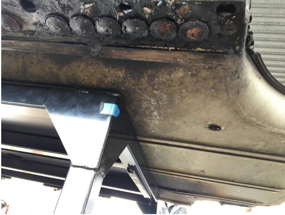
Burbank Inspection Photo 29: view showing right side front vents, after cover has been removed
