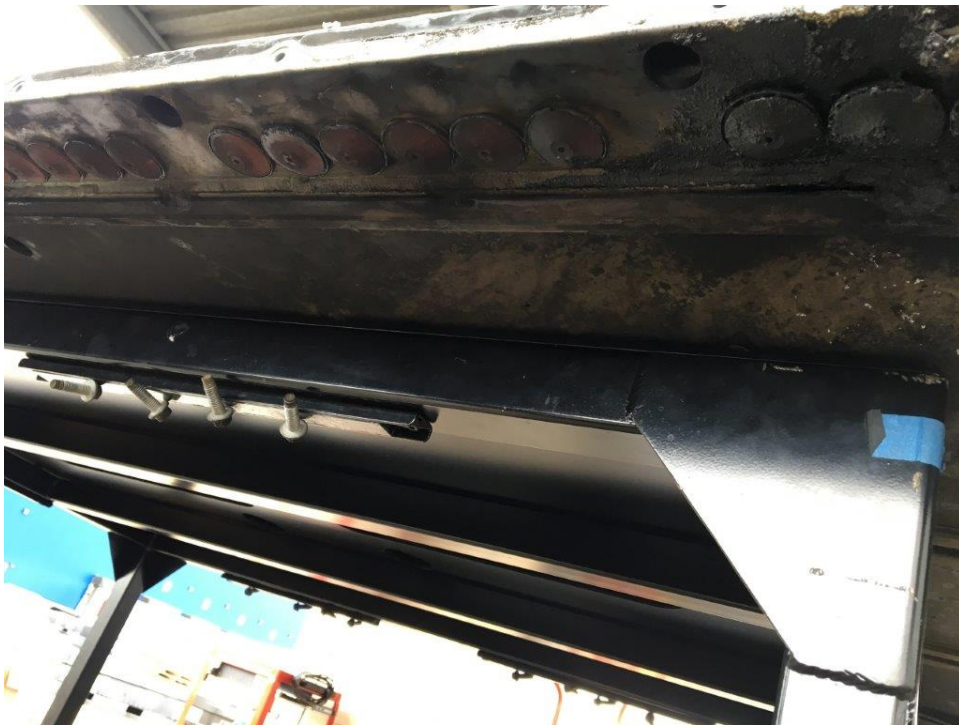
Burbank Inspection Photo 30: view showing right front middle vents, after cover has been removed
