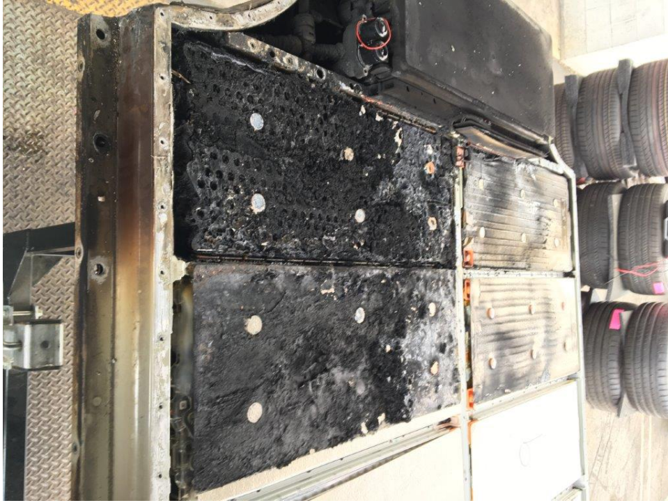
Burbank Inspection Photo 49: left front with covers removed and insulation for 11 to 14 removed
