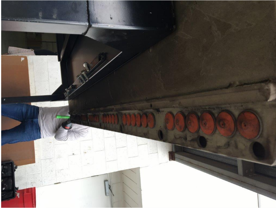
Burbank Inspection Photo 32: view showing right rear vents, after cover has been removed
