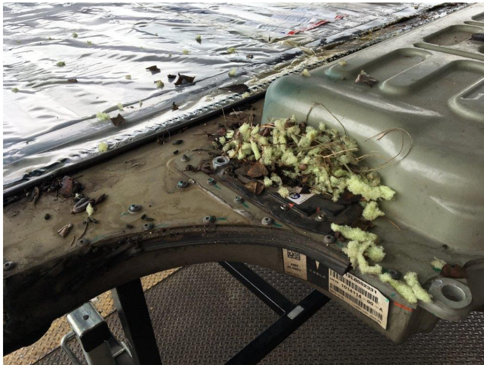
Burbank Inspection Photo 26: top left front battery pack as removed, showing rodent nest
