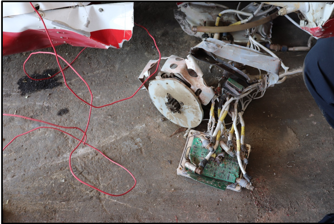
Figure 11: View of electric motor damage.
