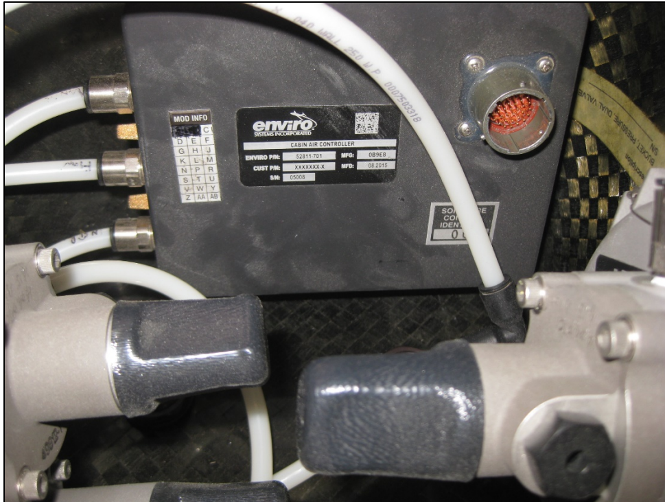
Figure 3 – Close up photograph of Outflow Valves and Cabin Pressurization Controller, as Received.
