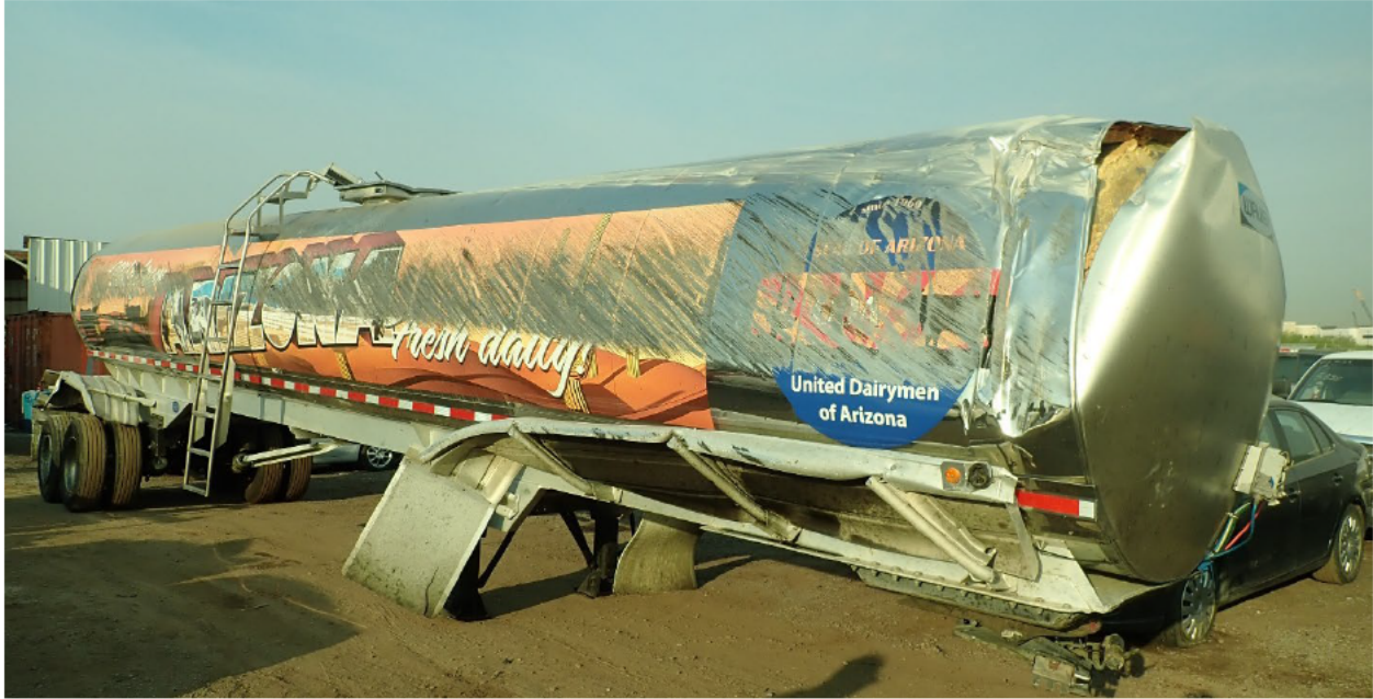
Figure 5 - The stainless front cap of the tank-trailer was partially detached from the rest of the stainless trailer cladding at the top, exposing the foam insulation beneath.
