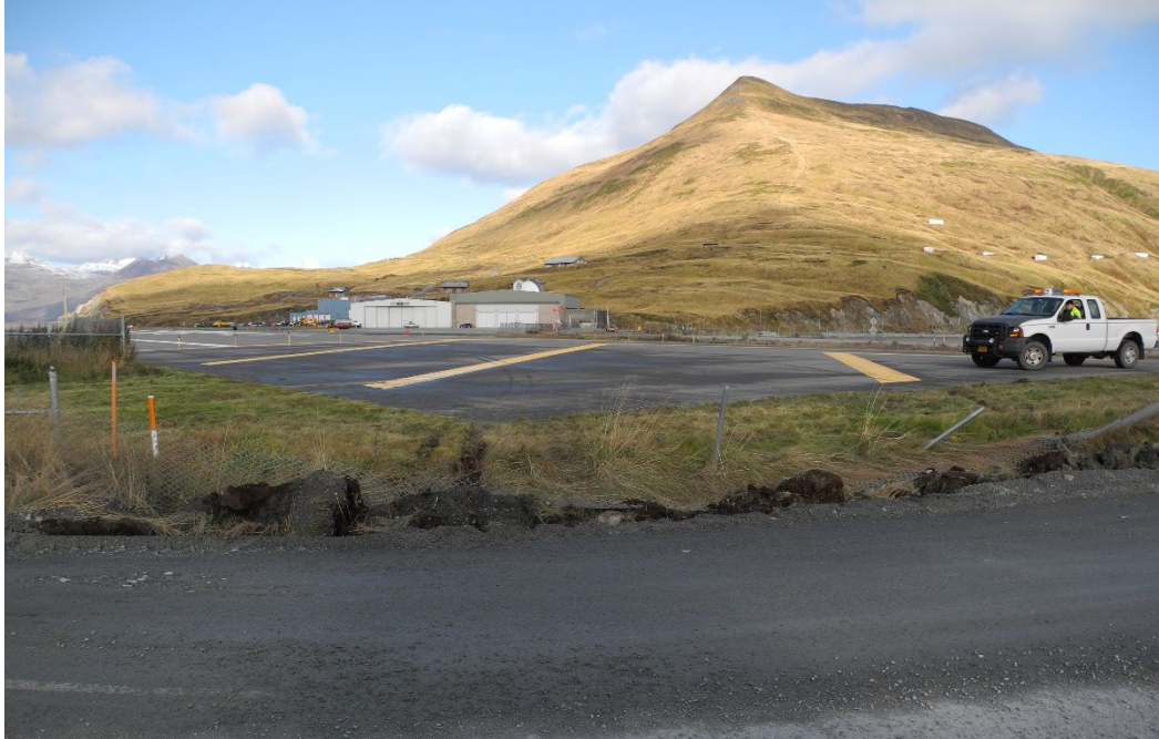
Photo 13. A postaccident view of the approach end of runway 31 showing the damaged perimeter fence and blast pad.
