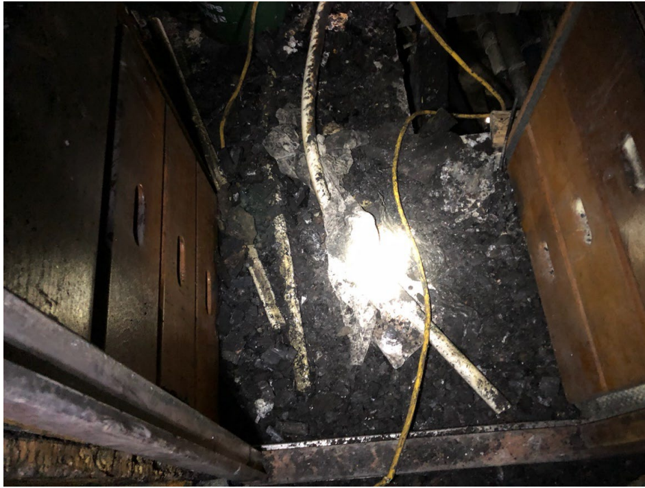
Image no.: 0254 Time: 1005 Description: Stateroom J floor area where welding machine was located.
