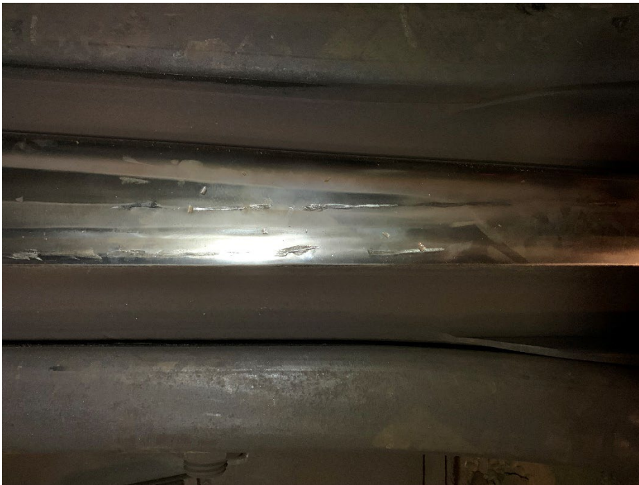
Figure 3. Wheel flange marks noted on the tread portion of the frog point at the C05 switch.
