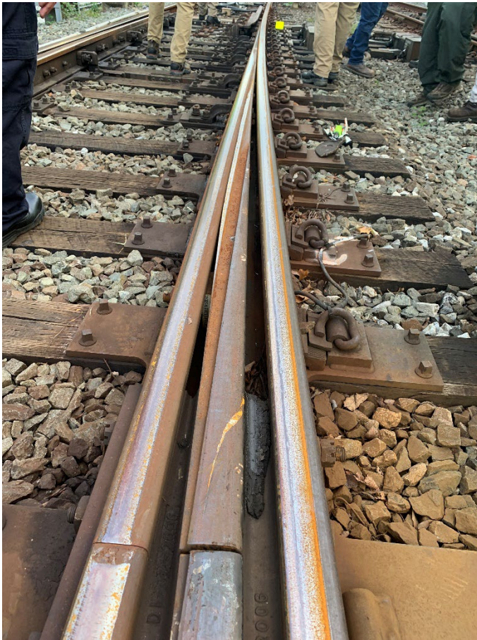
Figure 3. Wheel flange mark seen coming across the switch point near the heel of the switch in the 1A switch in the Arlington Cemetery station area.
