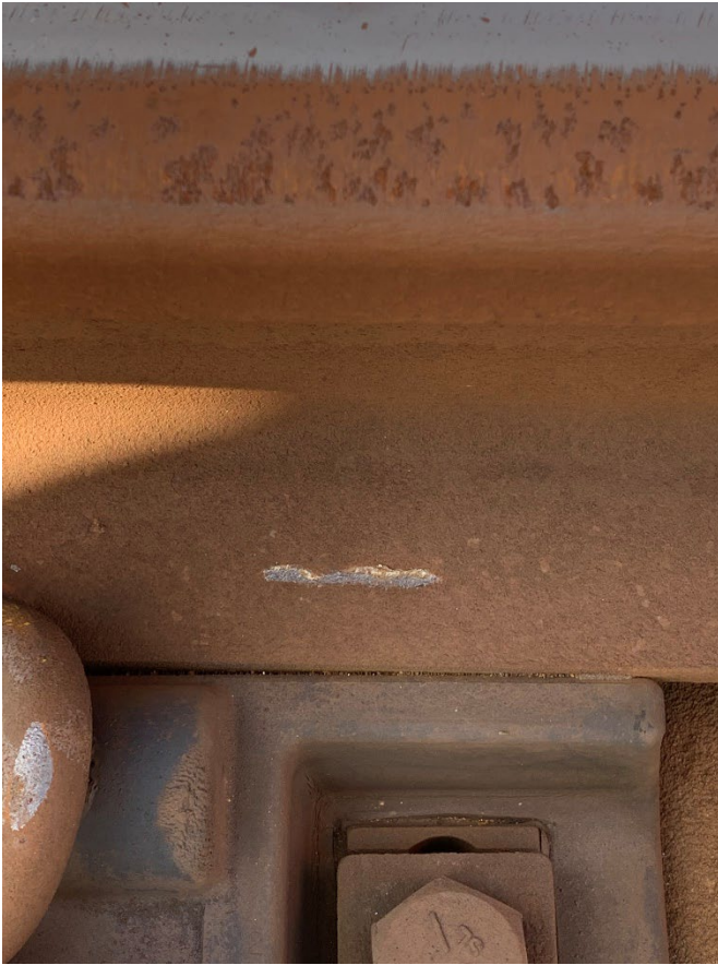
Figure 6. Corresponding wheel flange marks noted on the rail base in the G05 turnout.
