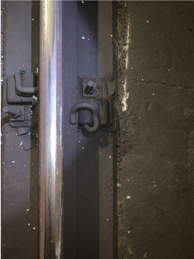
Figure 2. Corresponding wheel flange marks noted south of the frog on the concrete invert/tunnel floor near the C05 switch.
