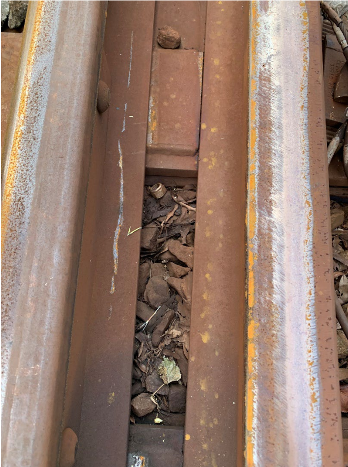
Figure 4. Corresponding wheel flange departure marks near the heel of the switch in the 1A switch in the Arlington Cemetery station area.
