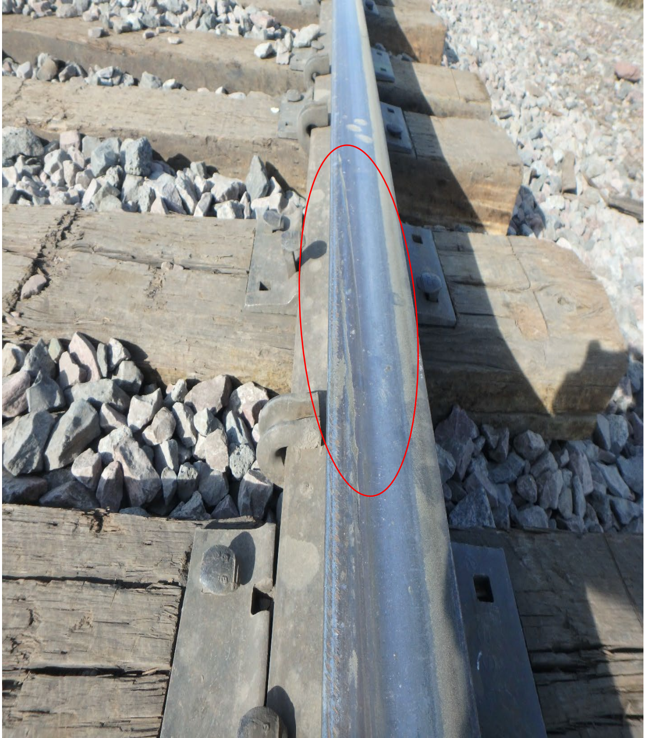
Figure 4- low side rail show wheel departure marks
