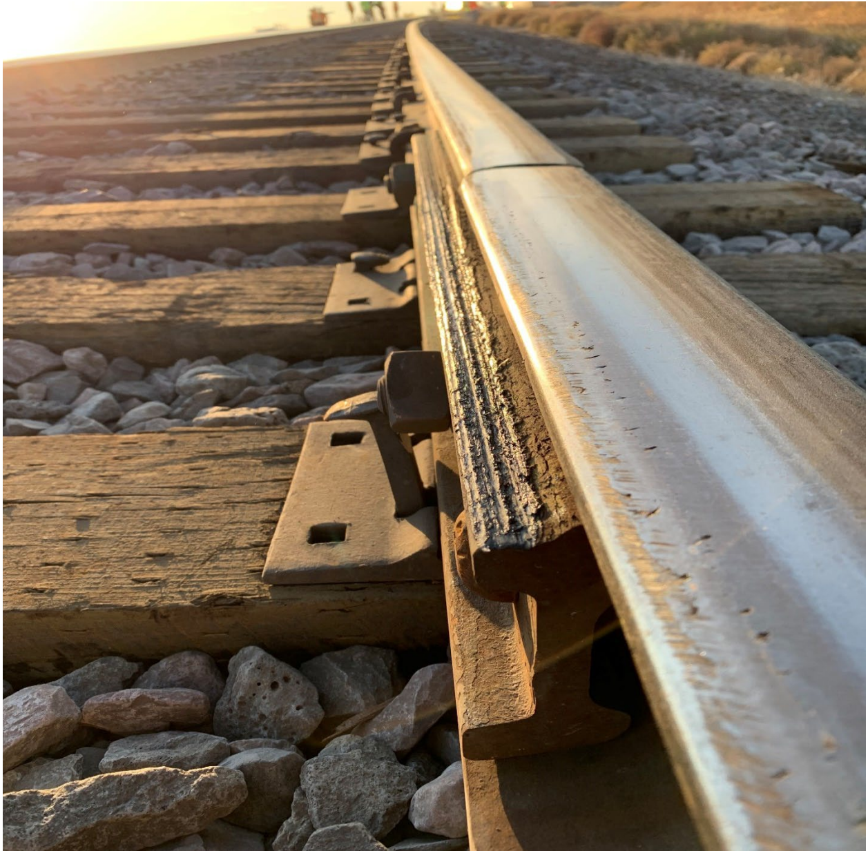
Figure 2- East low/north plug rail joint showing indication of wheel flange contact
