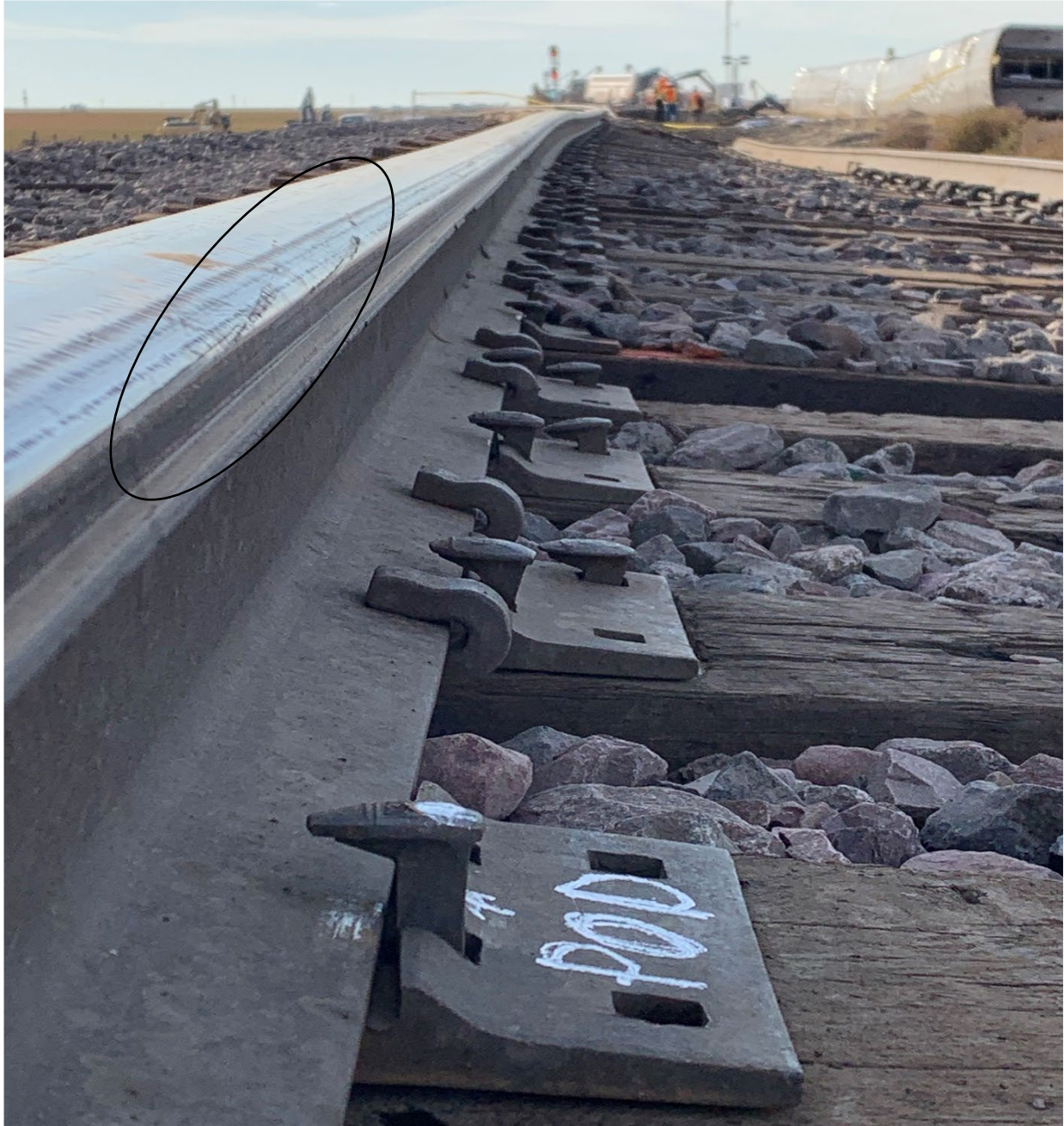
Figure 3- Point of Derailment looking west. High rail or south rail showing wheel departure marks
