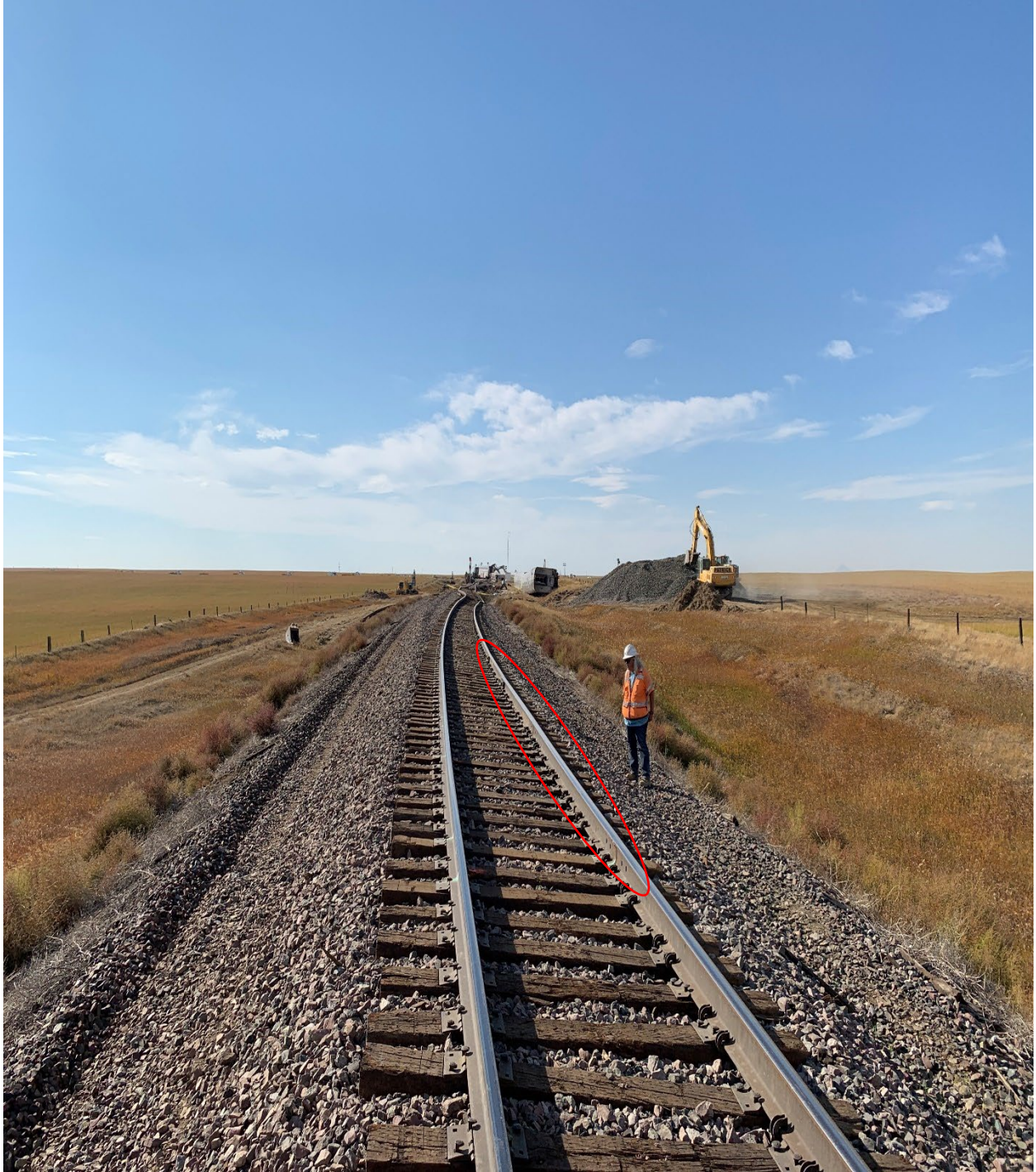
Figure 3- Photo of the in-track 19'6" bolted plug rail and two in-track welded 19'6" plug rails
