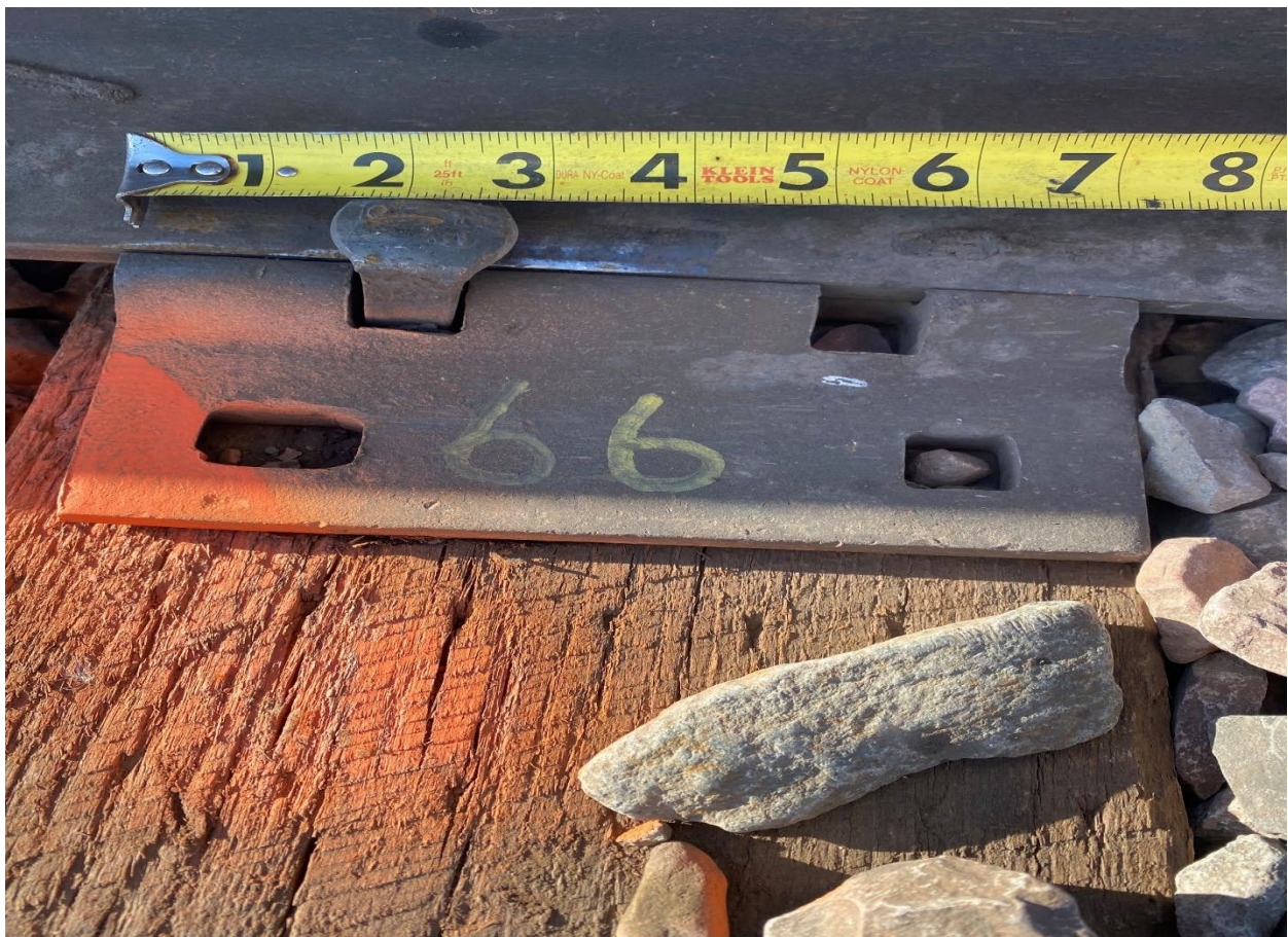
Figure 4- Photo showing longitudinal rail movement through spike.
